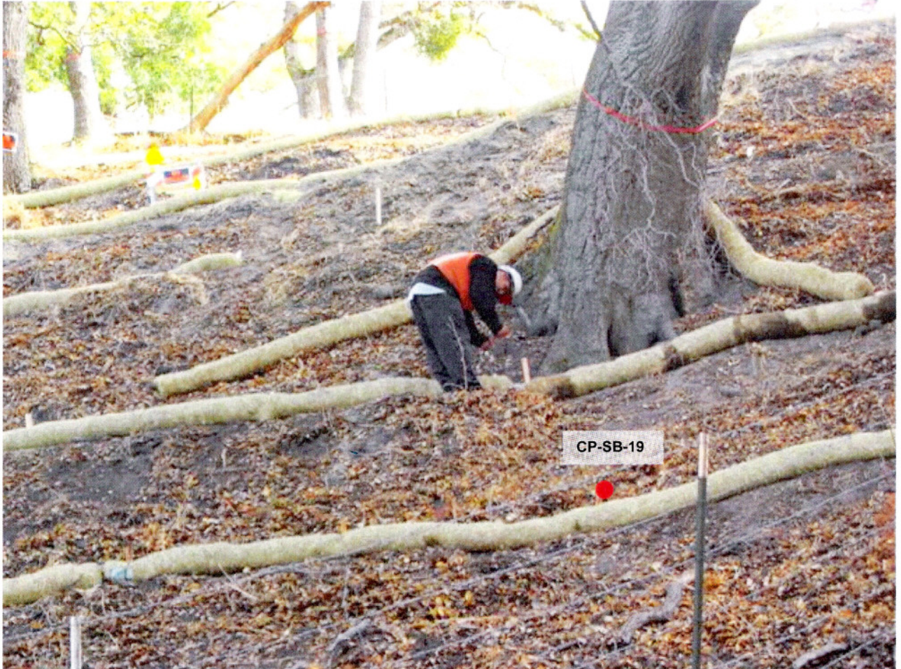
Photo 3 Steep 84-percent slope immediately below the pipeline release location, December 7, 2005.
