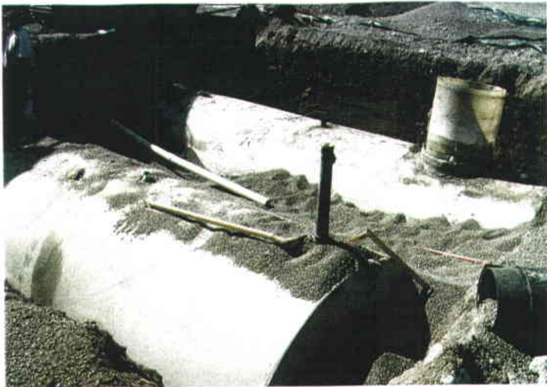
Photograph of underground storage tanks.
