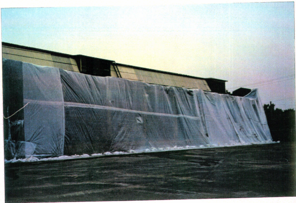
Photograph #5: East wall of the former Rifkin building after the non-hazardous bricks were removed.
