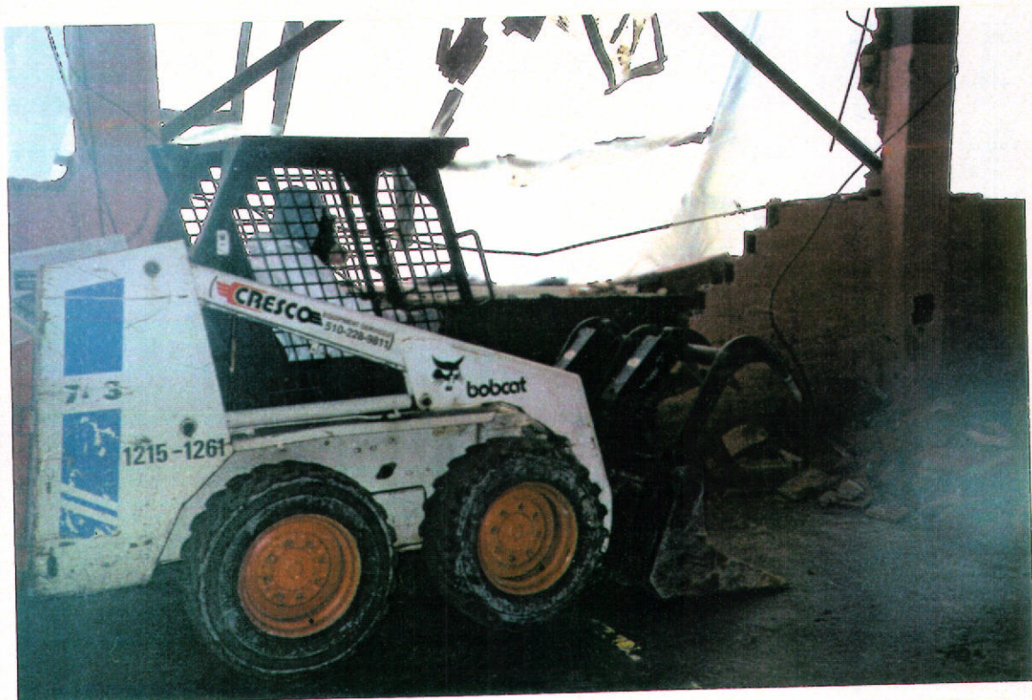
Photograph #6: Laborer in a bobcat removing hazardous bricks from the east wall of the former Rifkin building.
