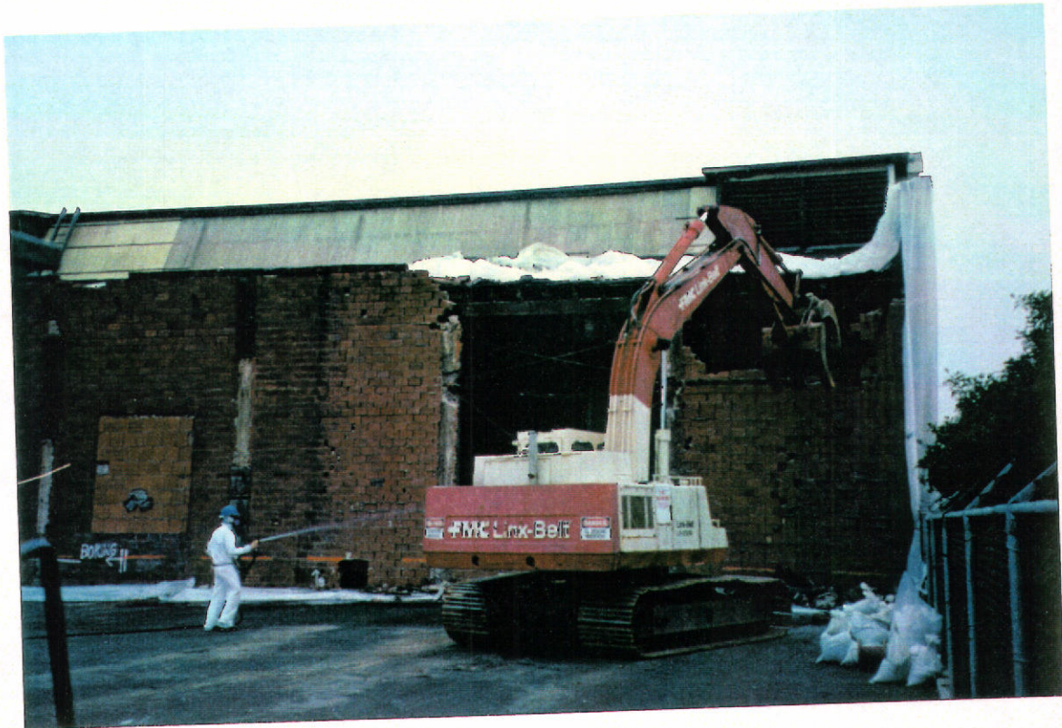
Photograph #3: Excavator demolishing the first bay of the east wall of the former Rifkin building. Note the laborer performing dust control in Level C personal protective equipment.
