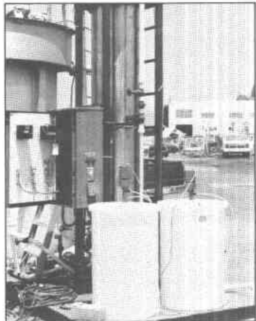
Fluidized-bed aerobic / anaerobic reactor modules, such as this 15 gallon per minute aerobic unit may be utilized individually, or in series, to remove organic contaminants from surface, ground and waste waters as well as soil.
