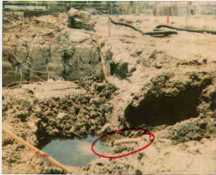
6/9/98 Waterhouse piping associated w/ WTS
