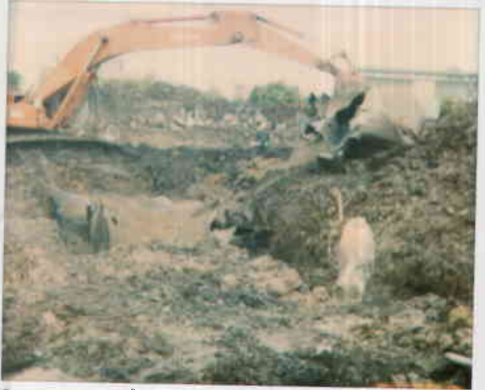
STID 5560 Former Waitinghouse 5/13/98 Tank #3 = ~ 5,000 gal.
