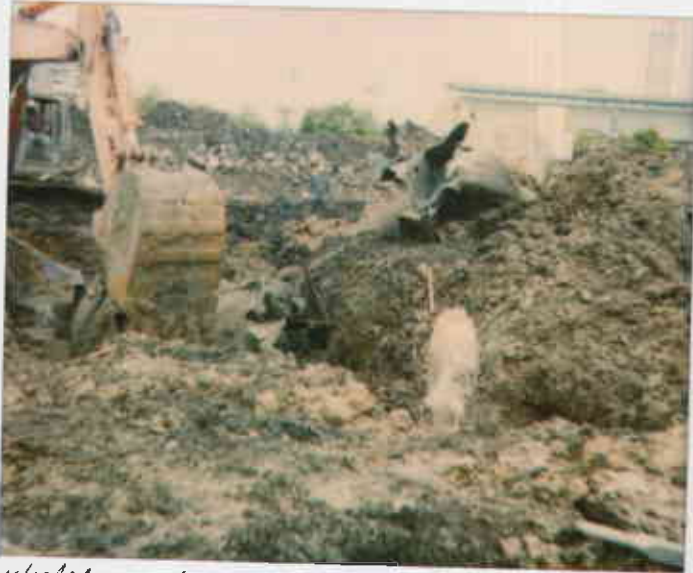
5/13/98 Former Waitinghouse Tank #3 ~ 5,000 gal
