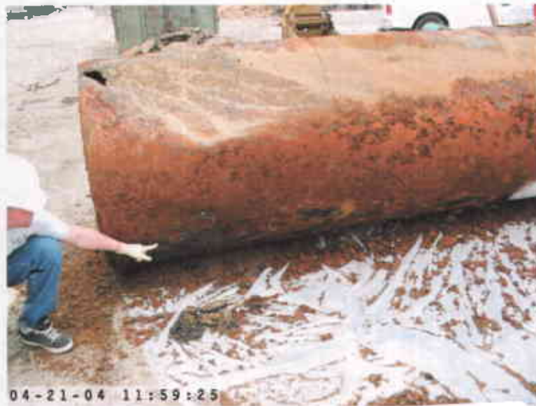
TANK REMOVAL RWESTON 4-21-04 MULTIPLE THRU GOING HOLES BOTTOM OF GASOLINE TANK 20957 BAKER ROAD CASTRO VALLEY
