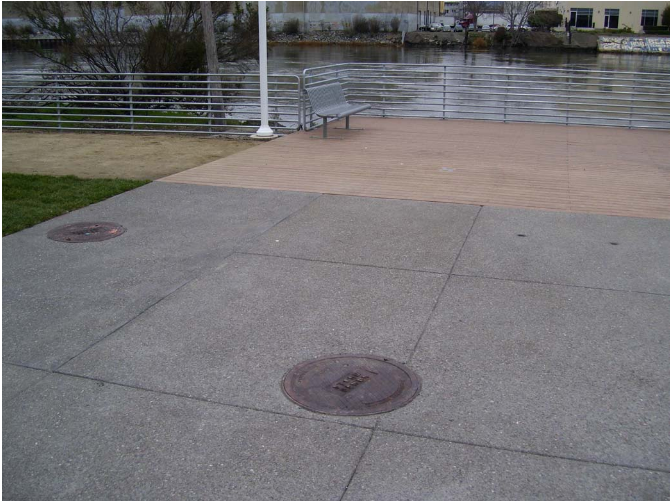
Photo 5 (MW-2). The photo above shows a close-up view of the anomaly (indicated by the two black spray paint dots in the right-center of the photo, near the interface of the concrete and deck surfaces) detected by the GPR. The anomaly was not detected while using the metal detector in the area. An “X” comprised of duct-tape is located on the deck, near the right central portion of the photo, and denotes the approximate location of MW-2 as measured off of the URS site maps when compared to the utility plan as-built (Sheet C-6.2). The photo was taken looking north-northeast.
