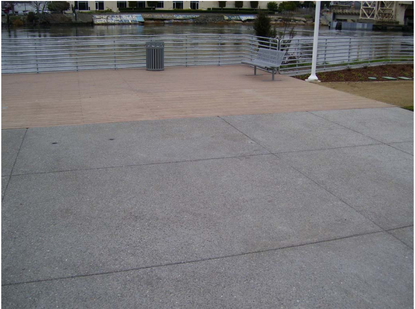
Photo 6 (MW-2). The photo above shows a second up-close view of the anomaly detected by the GPR near the interface of the concrete and deck surfaces (same feature shown in Photo 4). It is important to note that this anomaly appears to be located directly above the storm sewer mapped in the utility plan as-built (Sheet C-6.2) for the site. The photo was taken looking northeast.
