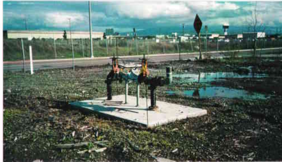
Photo 3. City water supply.
