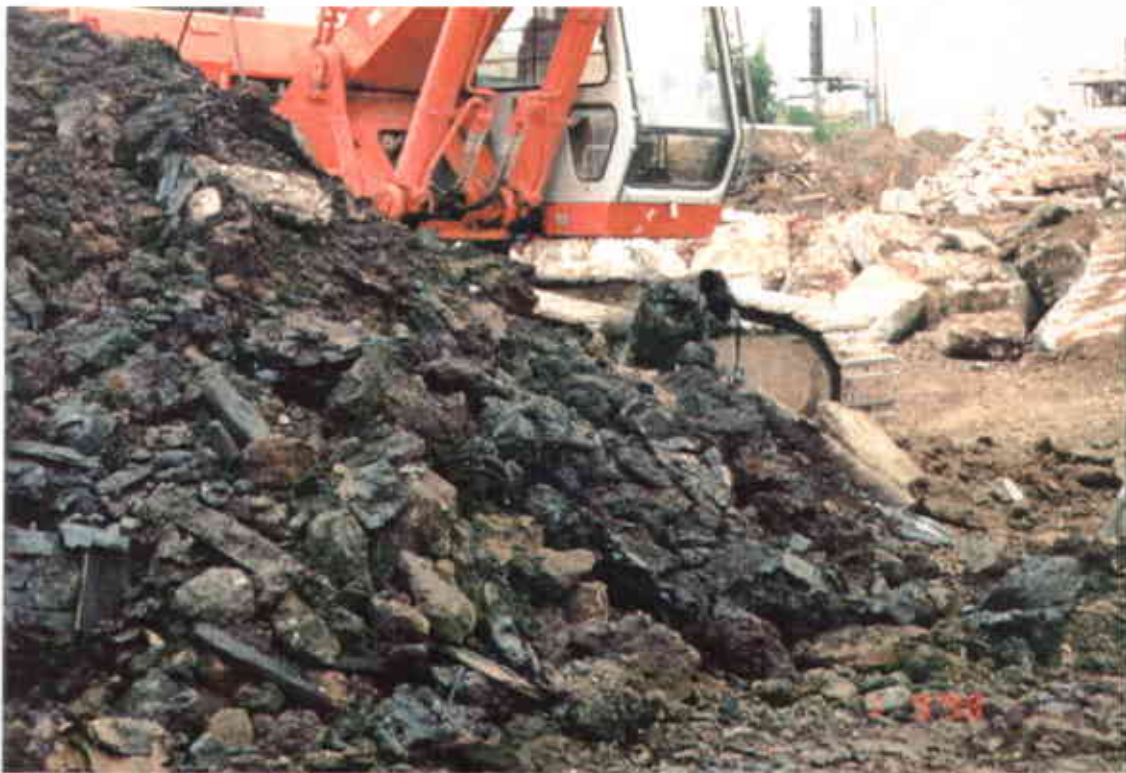
Photo 6: Contents of concrete vault located at the northern boundary of the former excavation
