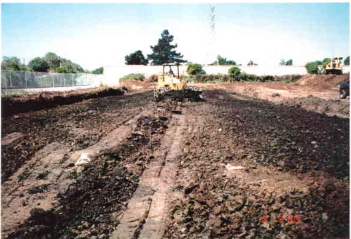
Photo 20: Compaction of the roofing shingles trench in the southern portion of the Site
