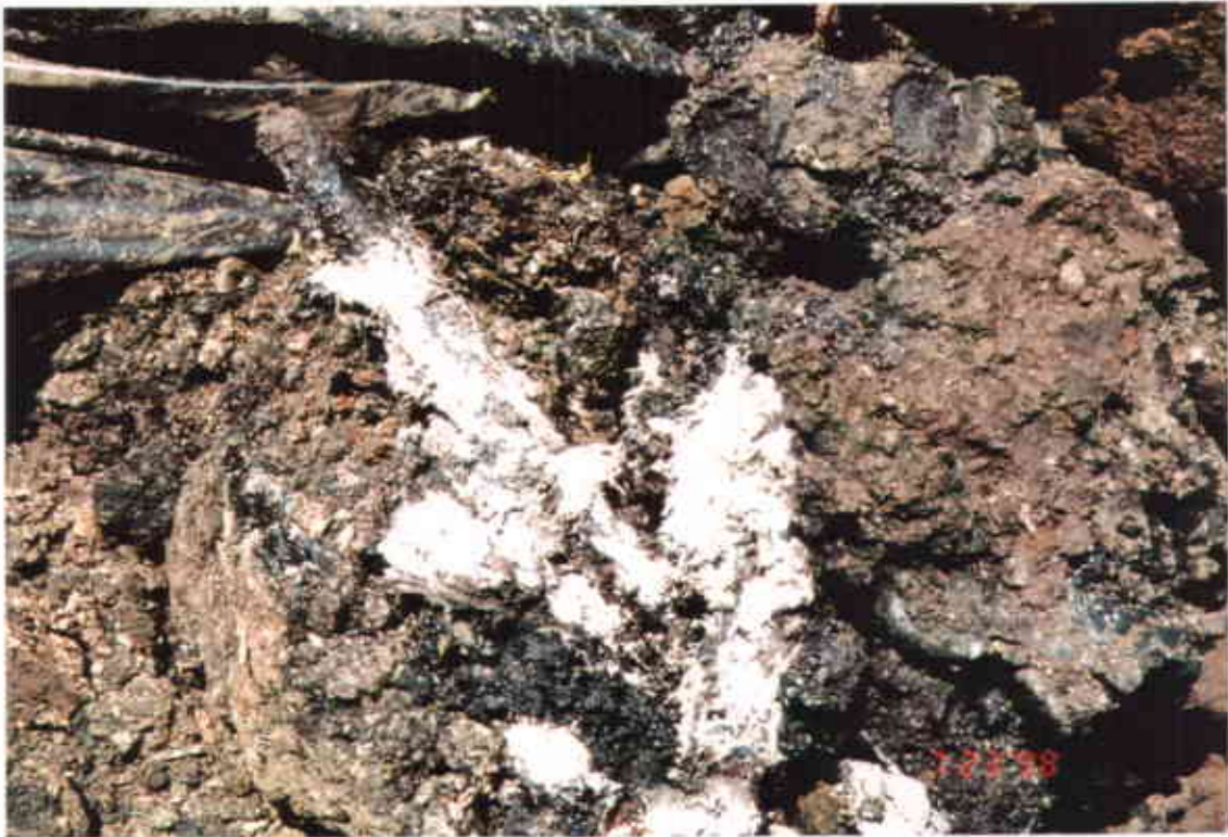
Photo 17: Pipes affected with asbestos containing material
