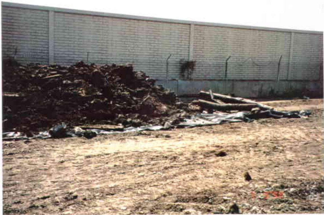
Photo 14: Contaminated waste and debris stockpiled in preparation for off-site disposal
