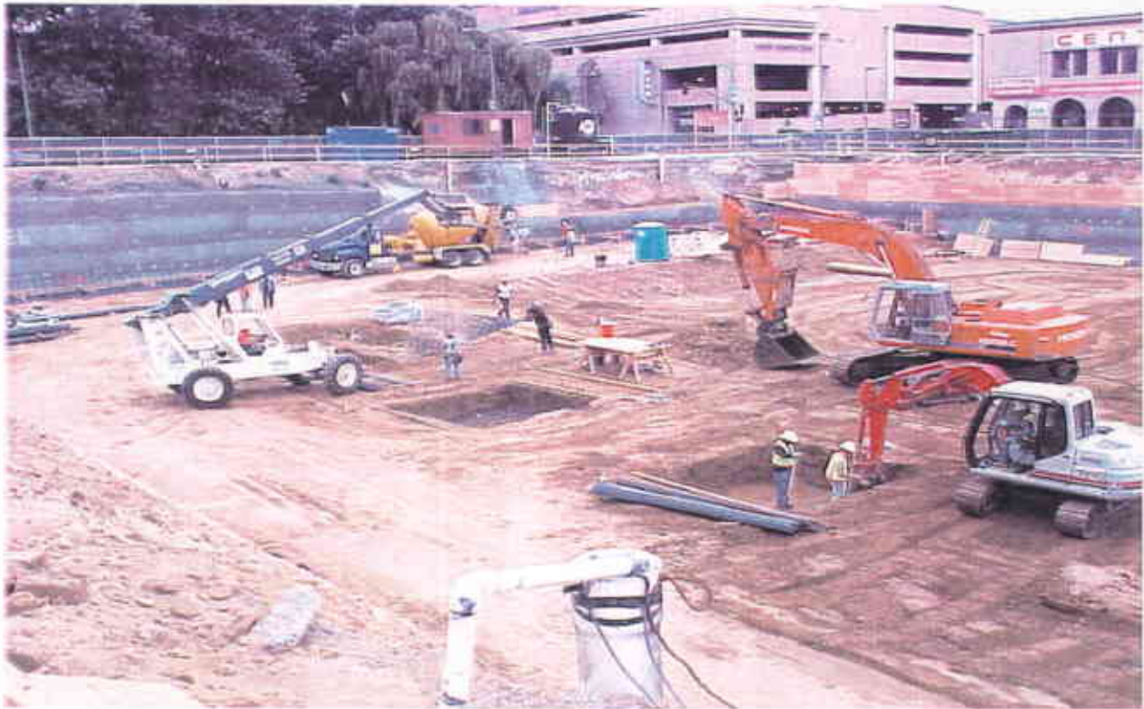
Photo 3 – Completion of Excavation with Groundwater Dewatering Well in Foreground (view to southeast)
