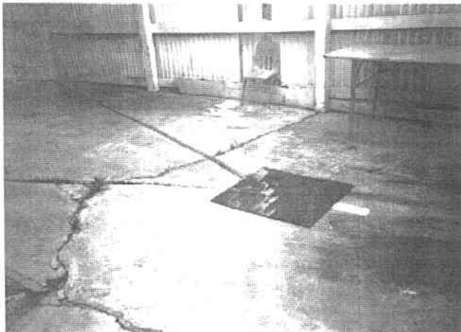
Picture 12: Covered grated drain previously used to transfer storm water to oil/water separator.
