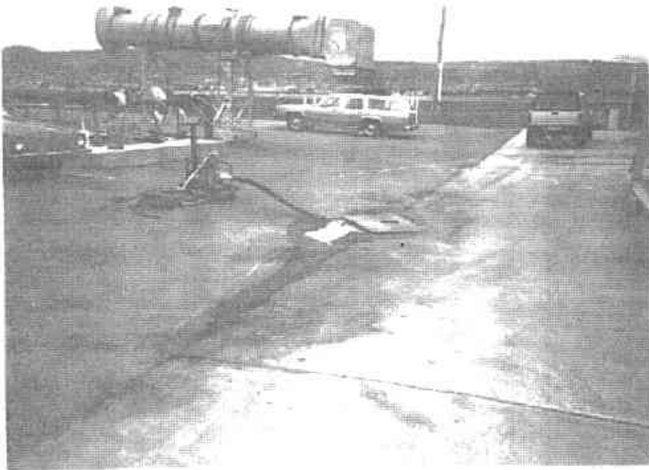
Picture 7: Pump and low area in asphalt/concrete parking lot where storm water collects.
