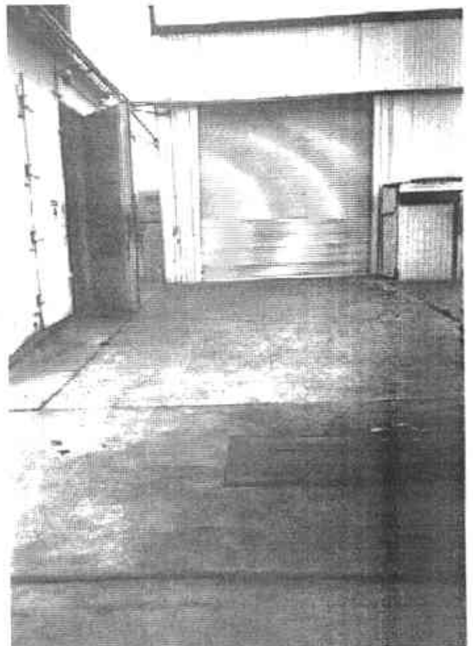
Picture 10: Covered grated drain previously used to transfer storm water to oil/water separator.
