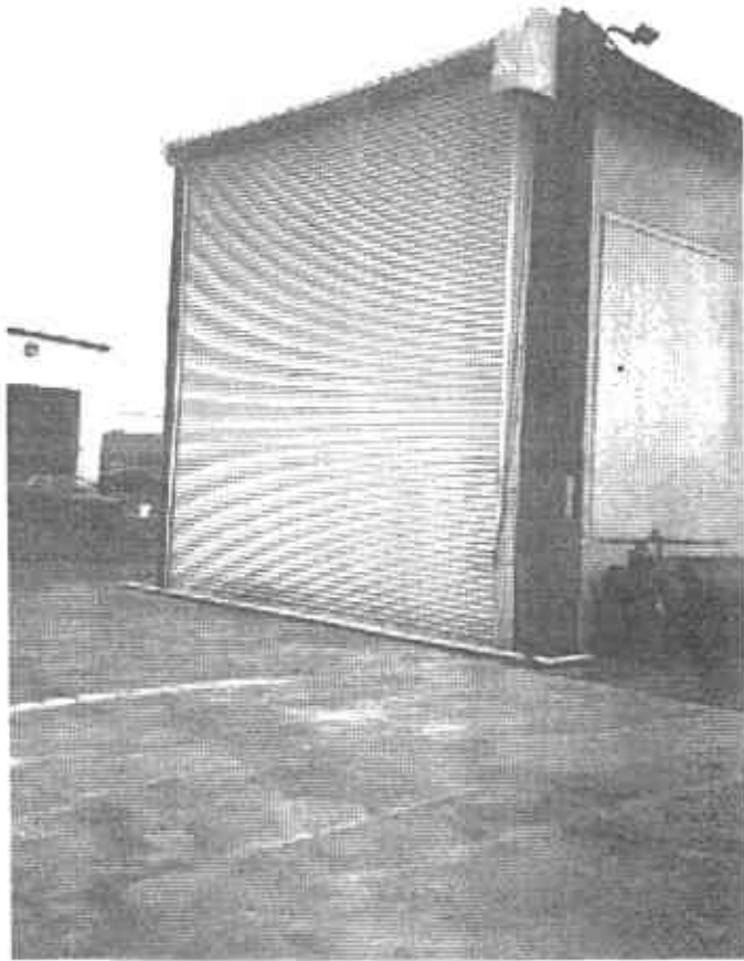
Picture 9: Engine test cell and PVC pipe for transferring storm water from the roof.
