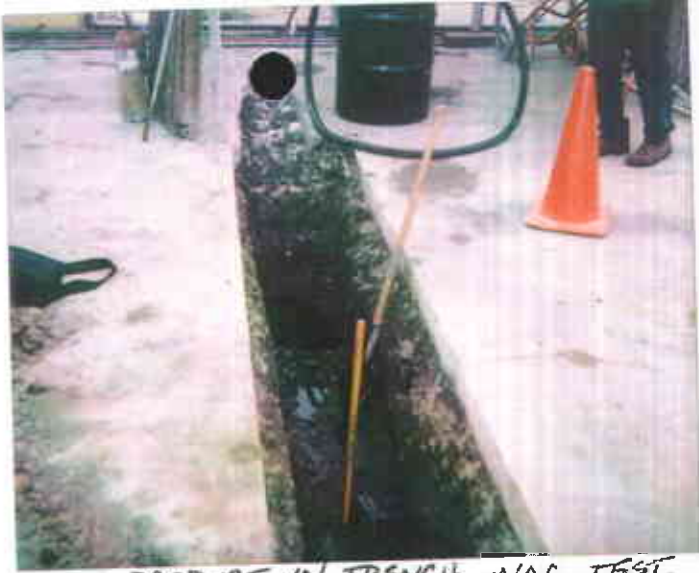
FREE PRODUCT IN TRENCH - NAC TEST 10/1/98 3:40P.M. - DHERMAN FACILITY
