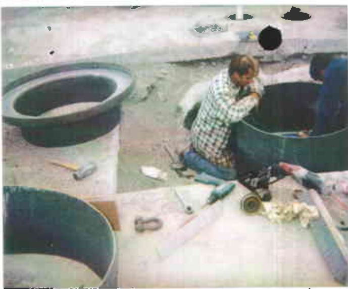
RETROFIT OF EXISTING 10K-GALLON UST NAC FACILITY - TEST CENTER 10/1/98 3:50P.M. - D. HERMAN
