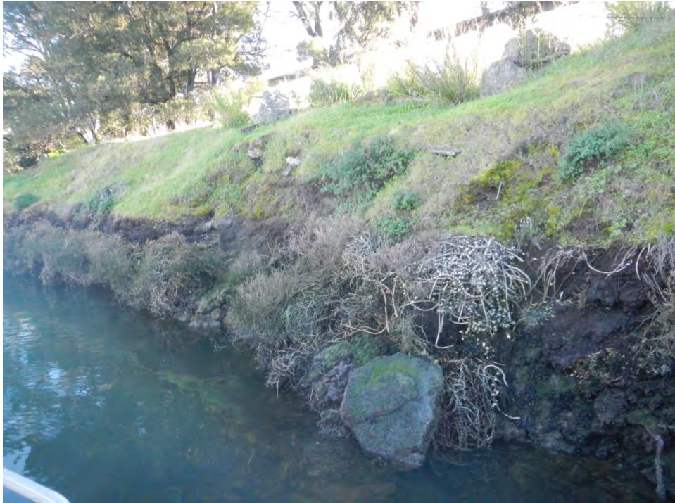
Photograph 37. Metal Shavings in Shoreline adjacent To SD-7 (January 12, 2015)
