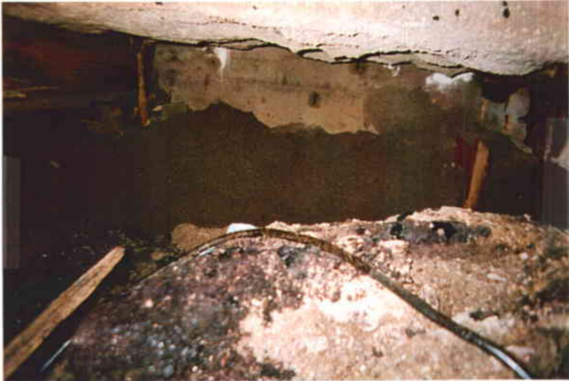
UST Vault Interior
