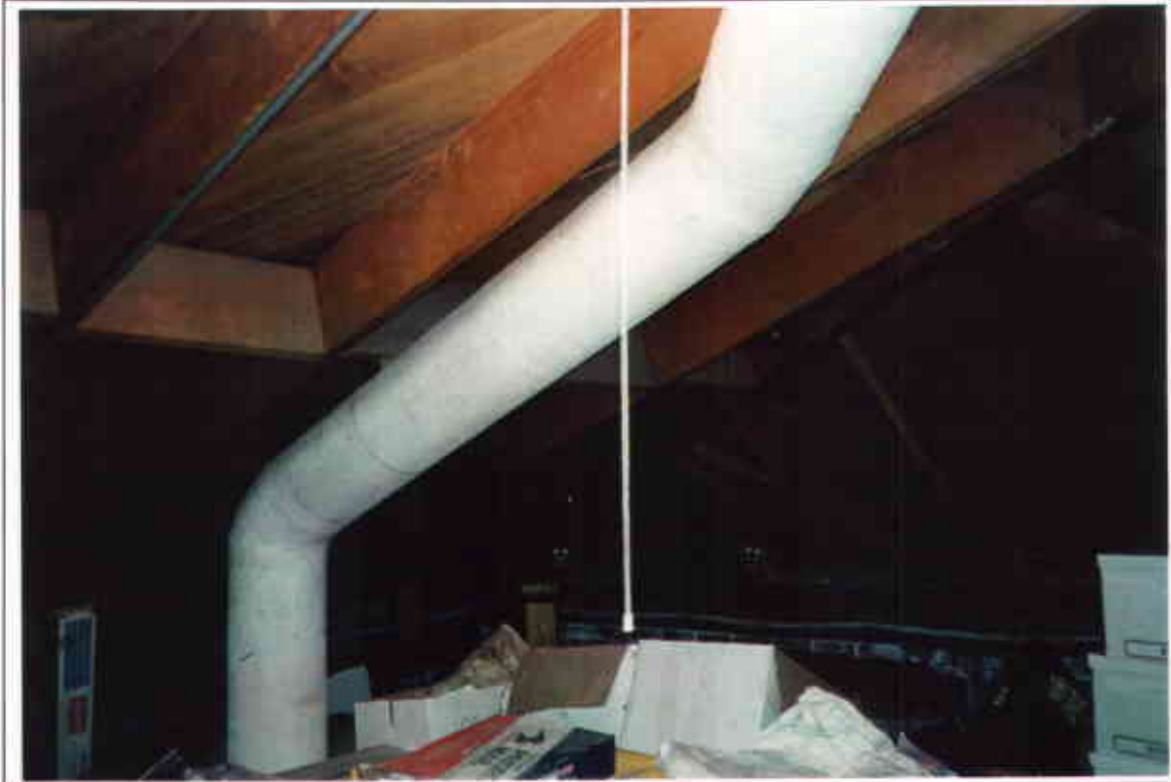
Photo 5: View of duct wrapping on the second floor of the office area of Thai Kitchen.
