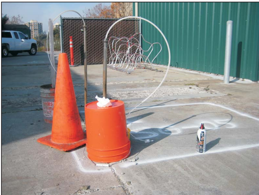
Photograph 14: Leak test at deep probe at SG-05.
