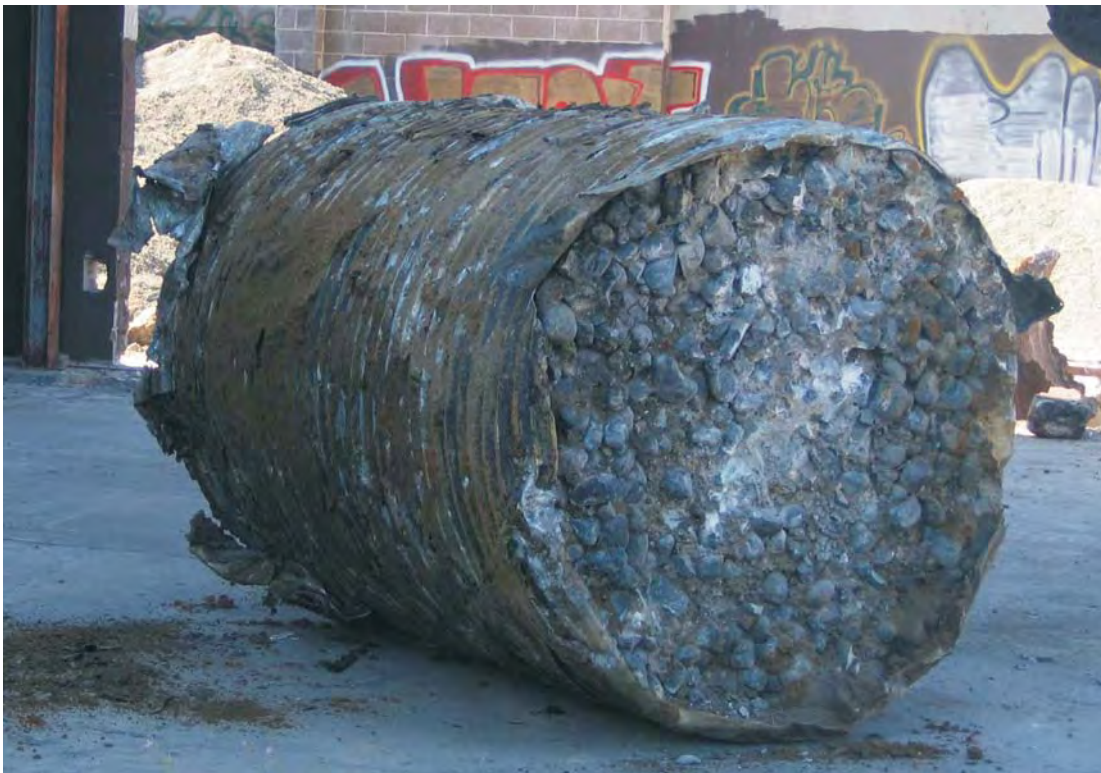
Photo 20: Base of Concrete Column after removal from Frog Pond - note cobbles imbedded in the bottom of concrete.
