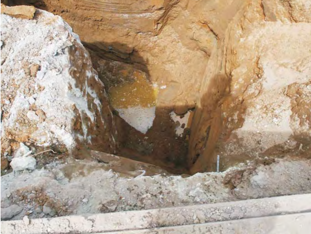
Photo 19: Groundwater seeping into excavation around Concrete Column.
