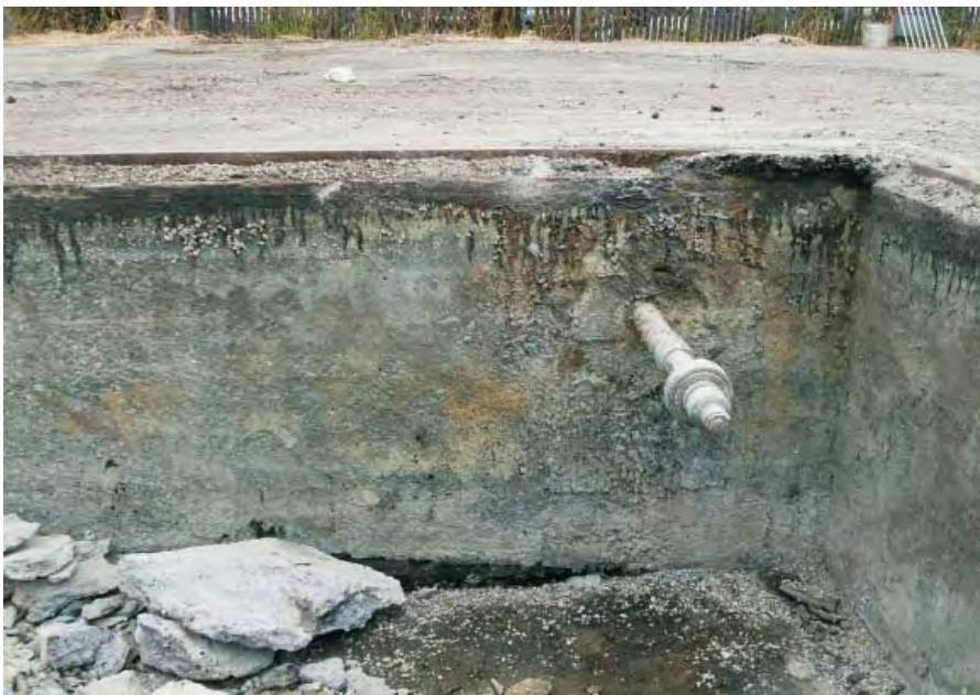
Photo 8: Metal pipe penetrating western sidewall of Frog Pond, sealed with screwed-in PVC plug.
