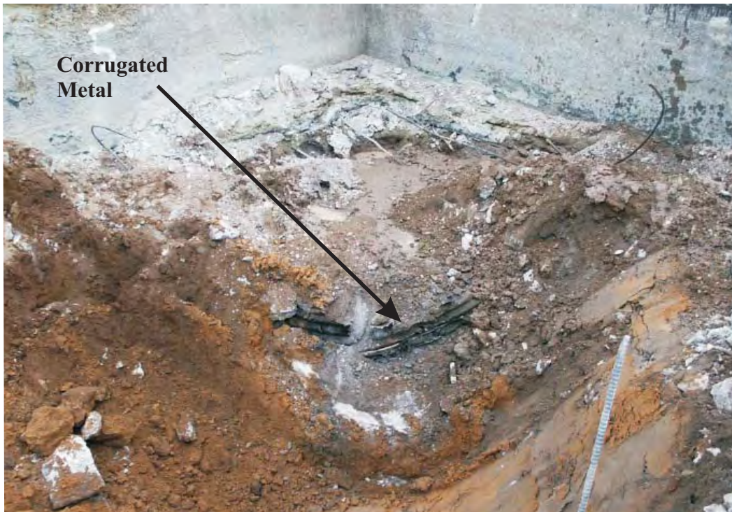
Photo 18: Corrugated metal sheeting surrounding Concrete Column (convex top broken away).
