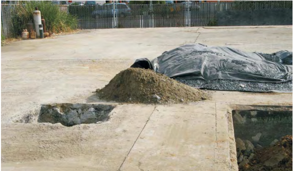
Photo 11: Western Vault uncovered (sand fill removed from vault stockpiled adjacent to vault).
