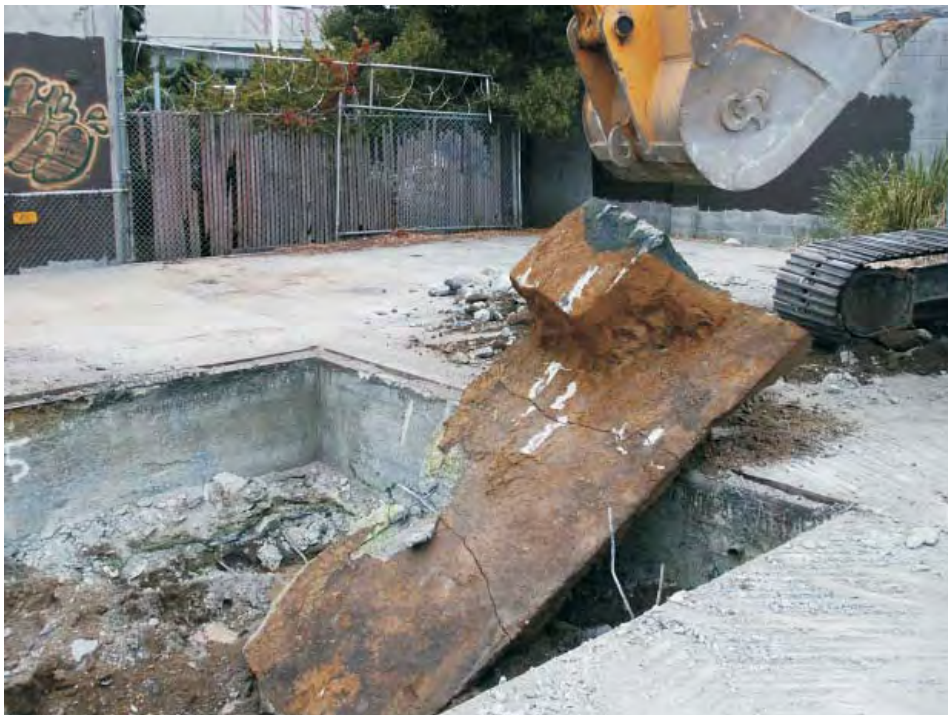
Photo 14: Concrete pad and sump removed from below the concrete bottom of Frog Pond (flipped over by excavator).
