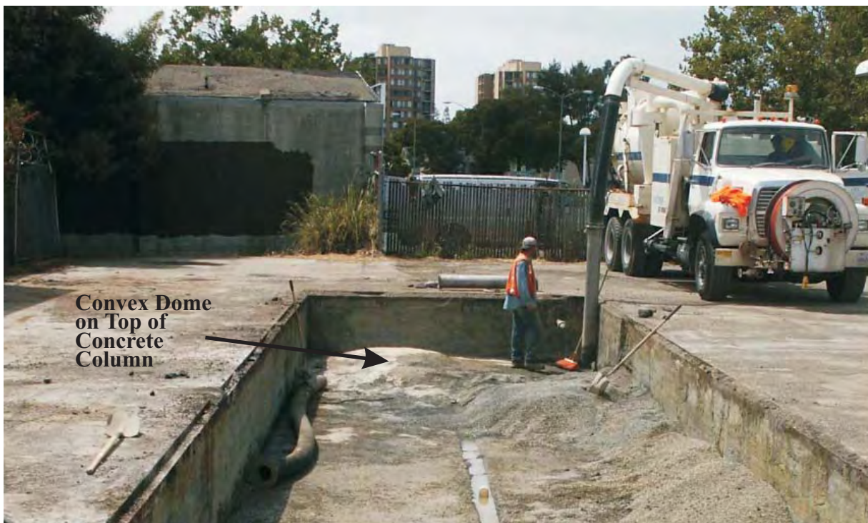
Photo 16: Concrete convex dome at the southwestern corner of the Frog Pond, corresponding to the top of the Concrete Column.
