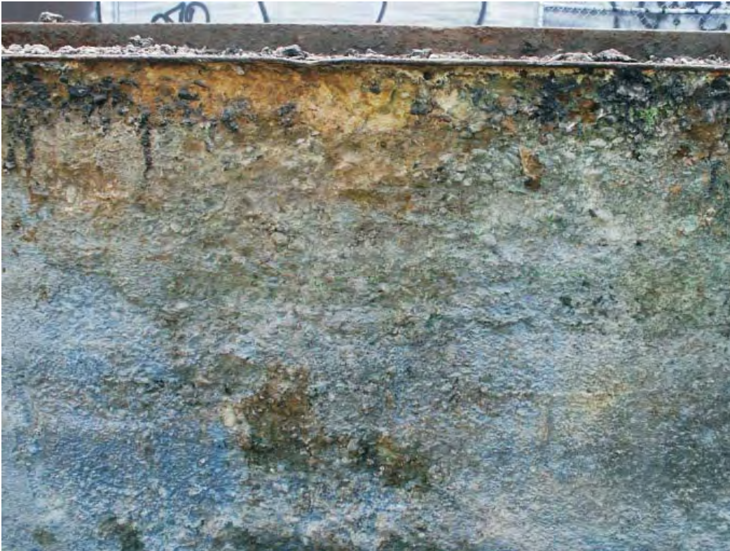
Photo 6: Staining on concrete on sidewall of Frog Pond.
