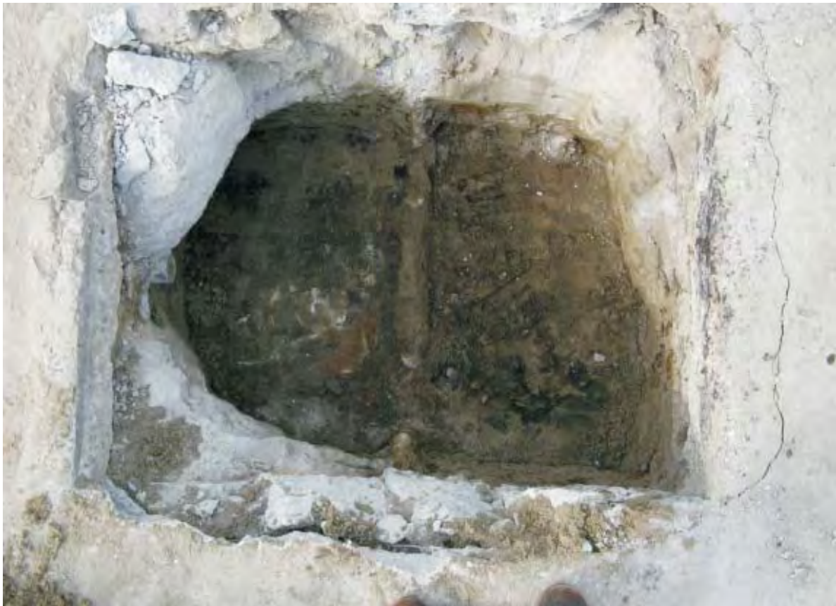
Photo 12: Interior of the Western Vault exposed (remnant of baffle in center; fiberglass bottom left of baffle).
