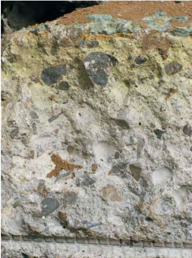
Photo 7: Evidence of permeation of chemicals through concrete (top of the concrete was on the interior of the Frog Pond).
