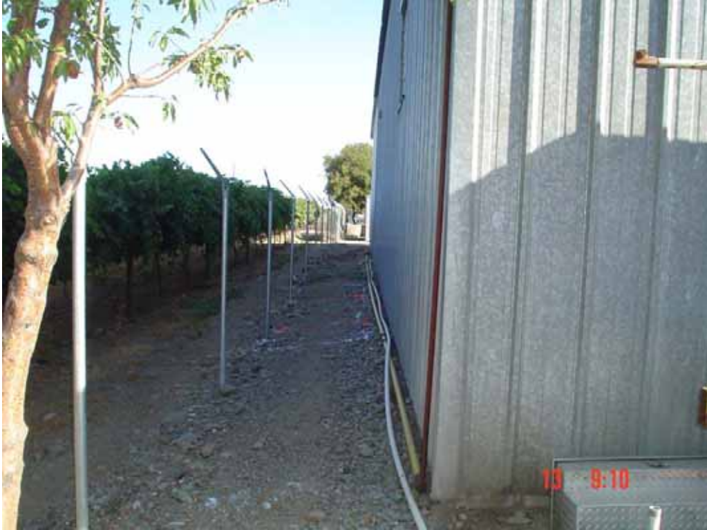
Above Ground Natural Gas Line (Yellow)
