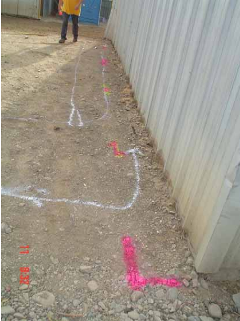
Below Ground Natural Gas Line Markings
