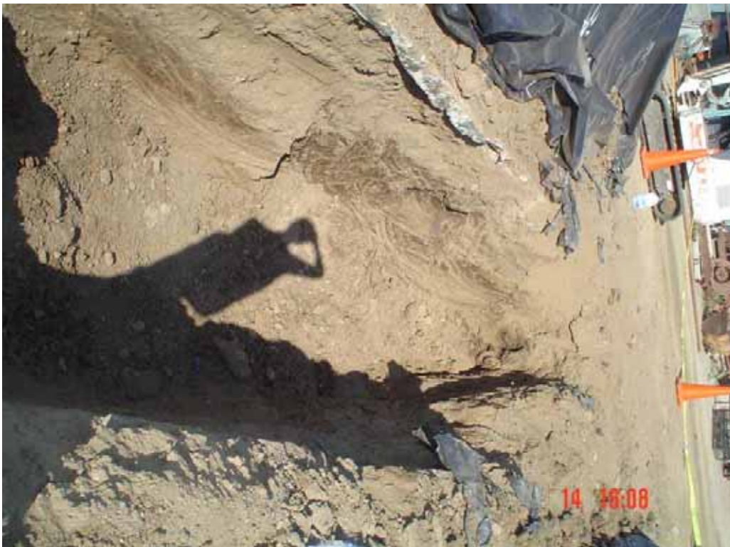
View of the Eastern Portion of the Excavation Area 4, after the First Excavation Phase (Rotated)
