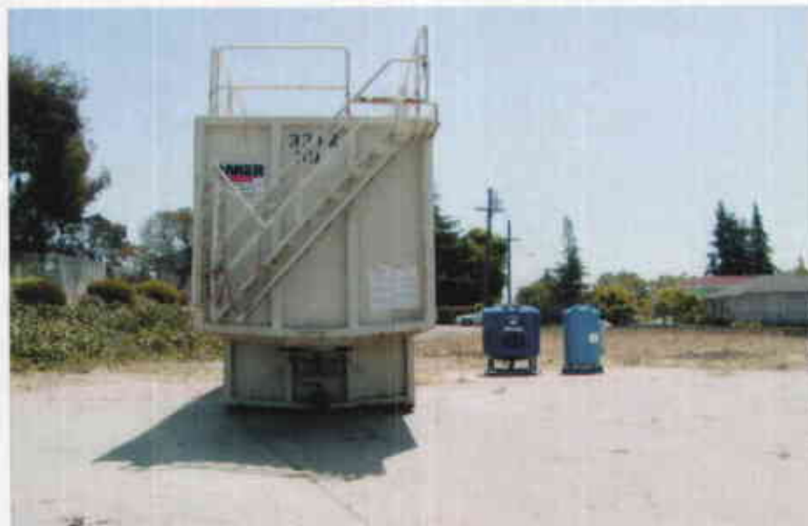
9. A view of the remediation equipment located at the former USA gas station (Parcel A).
