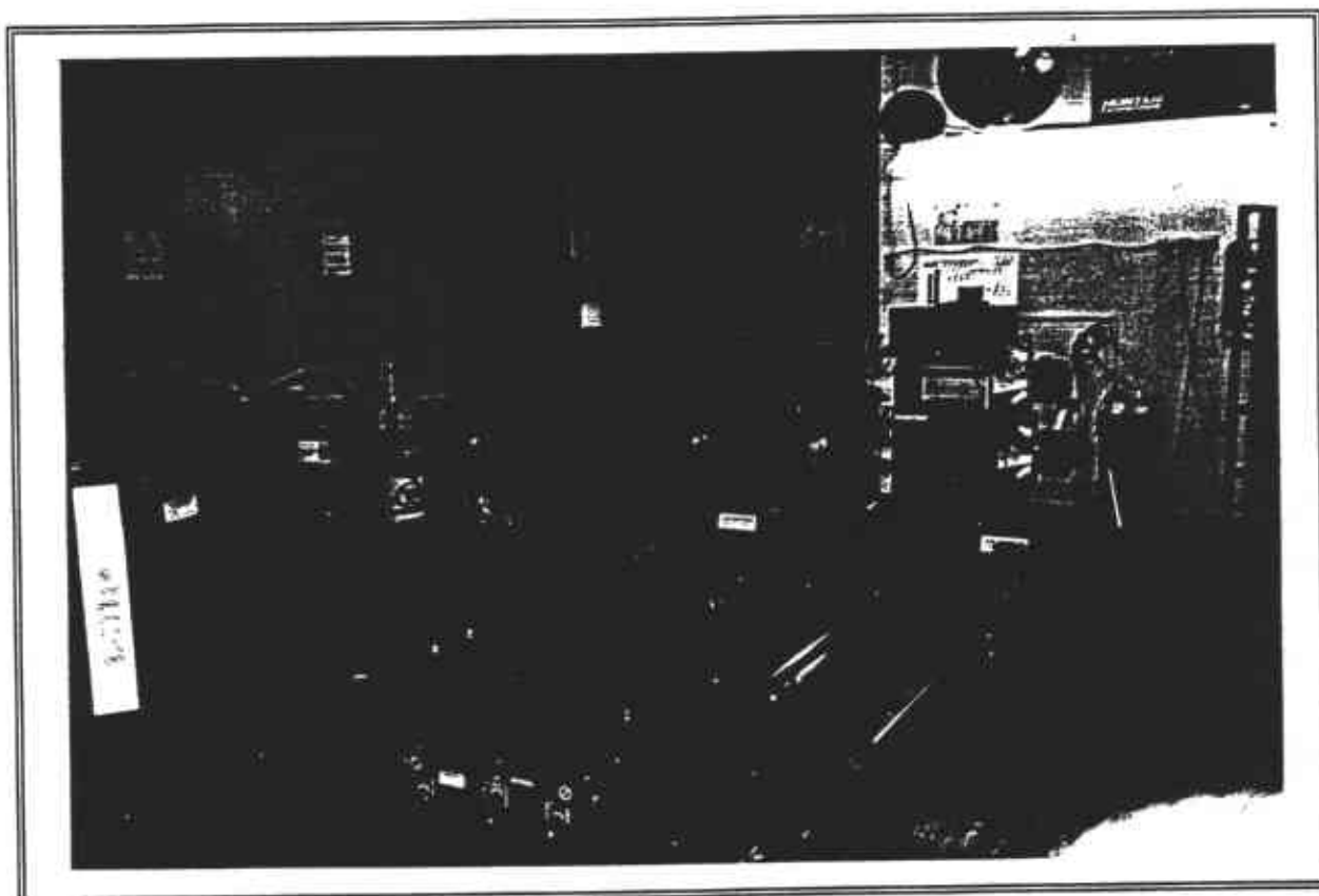
PHOTO 8: AIR COMPRESSORS AND ABOVEGROUND STORAGE TANK FOR HYDRAULIC LIFT
