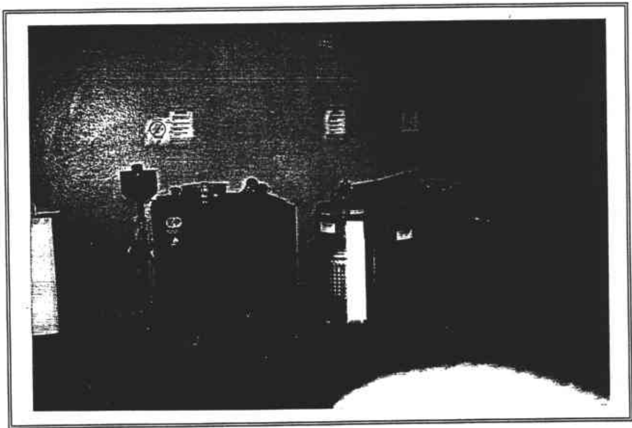
PHOTO 7: NEW OIL, USED OIL AND WASTE COOLANT STORAGE
