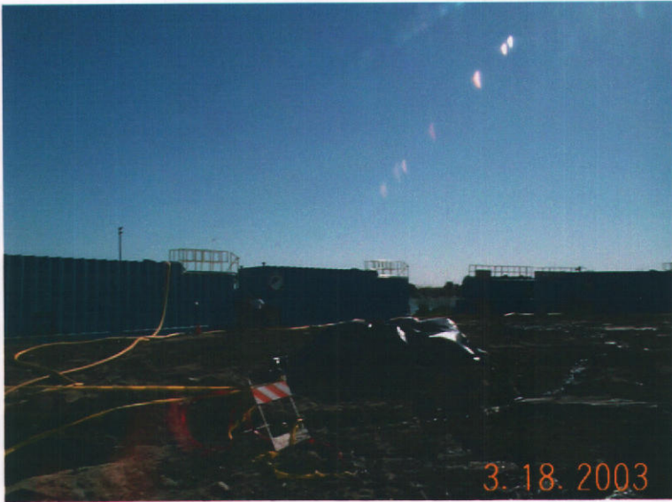
Baker tanks w/ extracted GW Seabreeze
