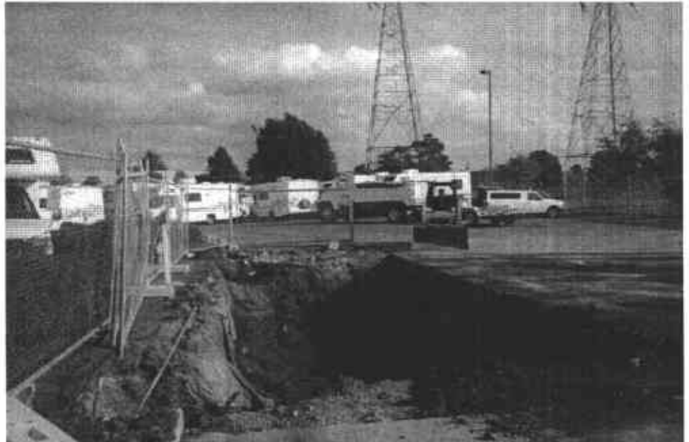
11. The excavation was partially backfilled to prevent groundwater from filling the excavation.
