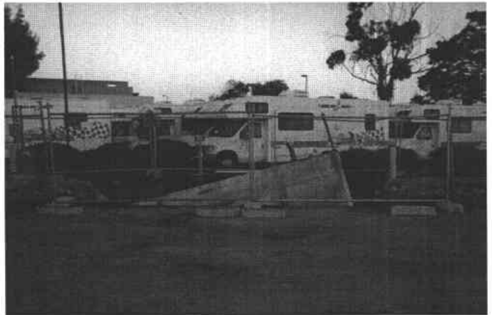
5. After the removal of the concrete pad and the upper layers of soil, the tank floated up. Groundwater was present at 4 feet below ground surface.
