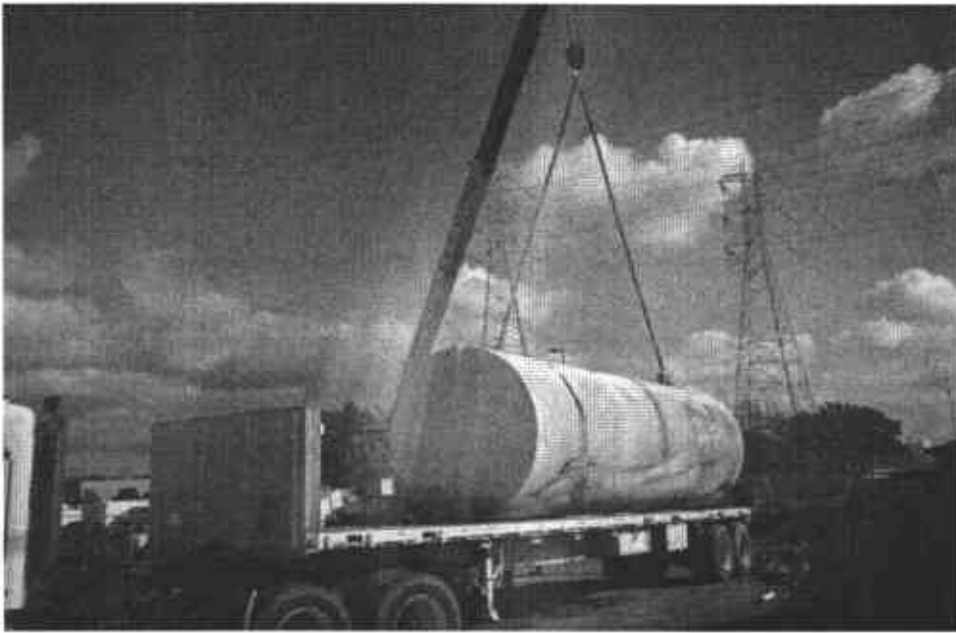
10. Tank is loaded onto a flatbed truck for transport to the disposal facility.
