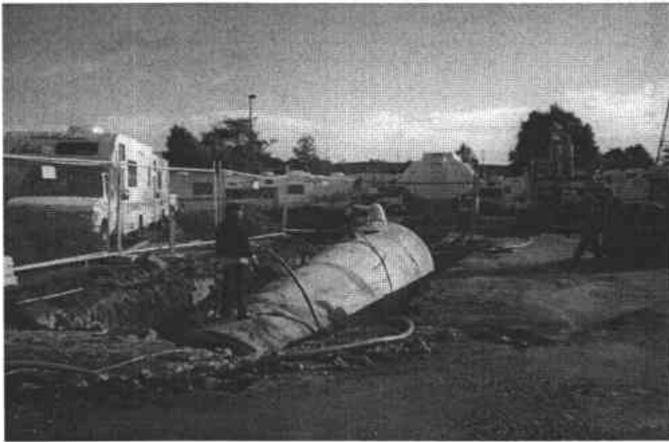
7. The liquid inside the tank was pumped out. The tank was rinsed with Simple Green and water in order to remove the explosive vapors.
