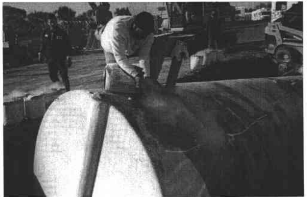
8. 600 pounds of dry ice was added to the tank. The dry ice pushes out all the oxygen and explosive vapors making the tank safe for removal and transport.
