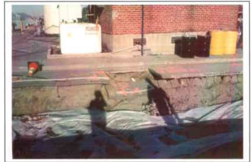
Photo 20. Undermined asphalt is falling into excavation pit.
