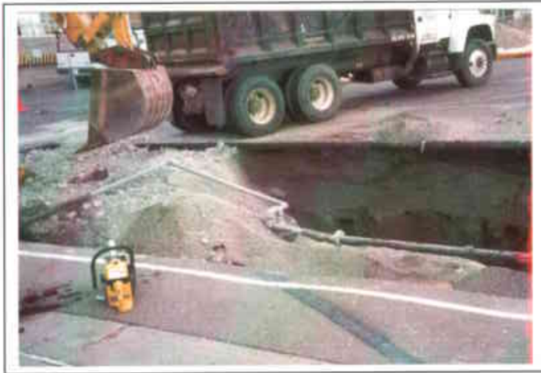
Photo 5. Excavated pea gravel being transported to stockpile while exposing bilge and vent piping located above tank. View towards east
