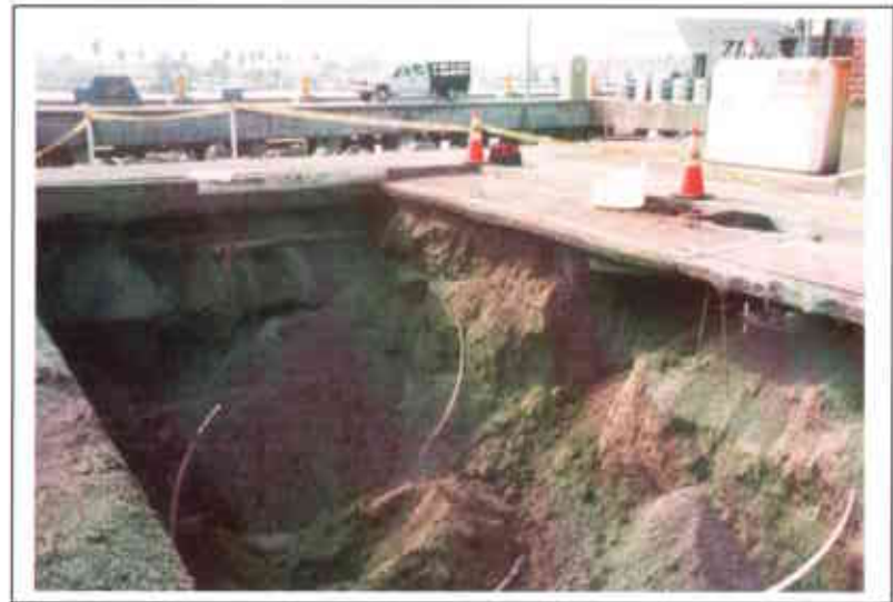
Photo 14. Northwestern and southwest sides of excavation. No water intrusion observed although immediately adjacent to bay.
