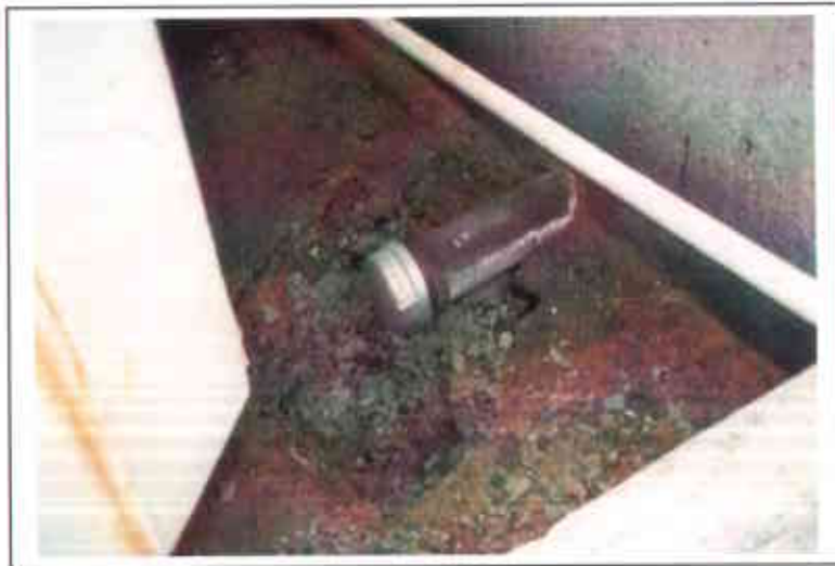
Photo 30. Detail of capped oily waste pipeline leading from Building 44 to tank. Located on southwest side of Building 44.
