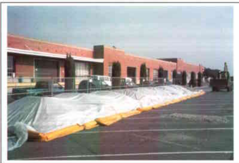
Photo 15. Eastern view of stockpile of excavated pea gravel. Material was excavated from east side to west side. Pea gravel was stored respectively from north to south side of parking lot.
