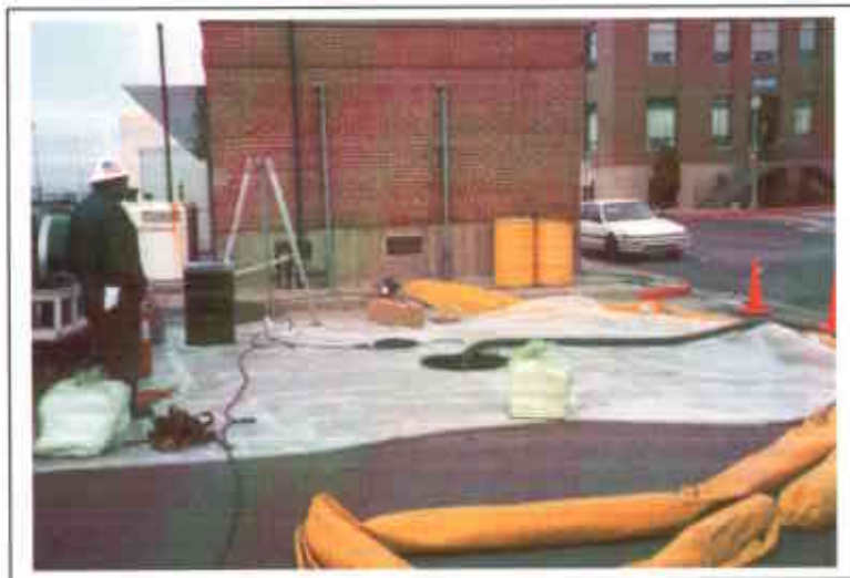
Photo 3. Set up for confined space entry into underground storage tank for cleaning.
