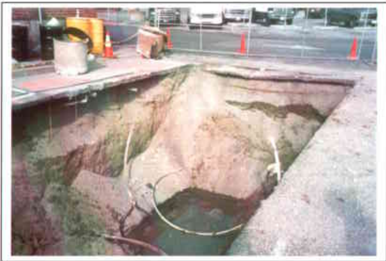
Photo 13. Northeastern and northwest sides of excavation hole after tank was pulled. Shallow groundwater intrusion into excavation.
