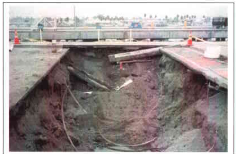
Photo 16. Curb on southwestern side fell into excavation.
