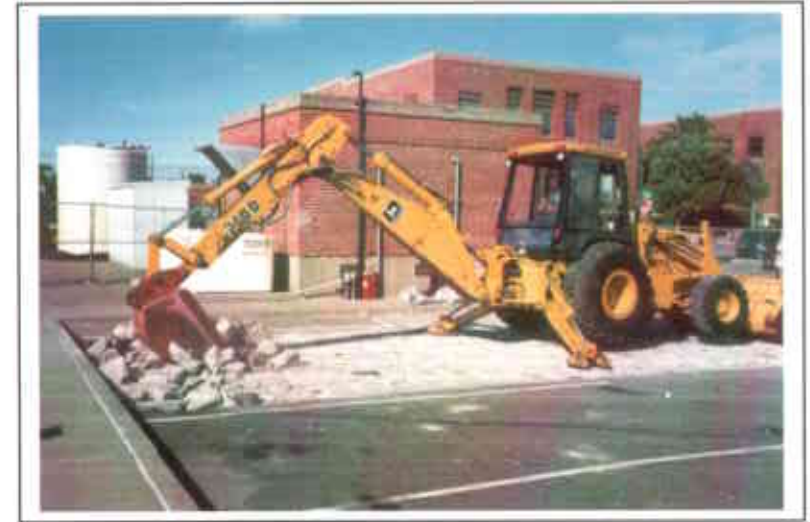
Photo 4. Removal of concrete from surface after high-pressure cleaning of tank before excavation.
