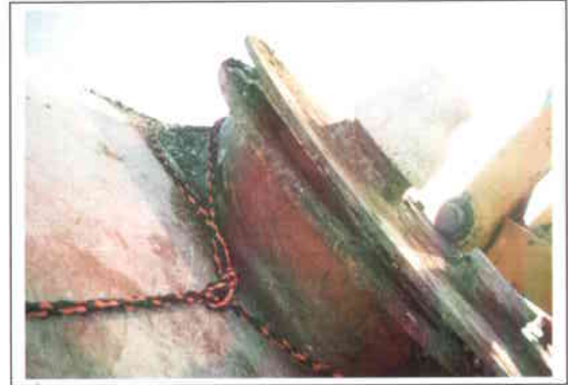
Photo 10. Detail of unbolted tank access for pipelines.
