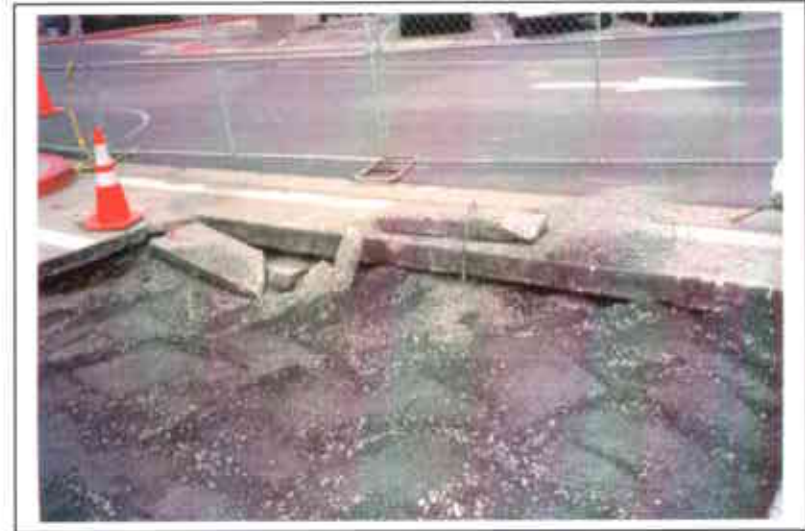
Photo 29. Detail of undermined gutter on east side of excavation due to vibration from compaction process.
