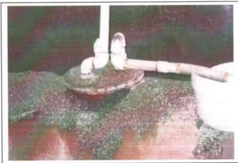
Photo 7. Detail of manhole from previous picture. Note the approximately 2-inch gap between hole and cover.
