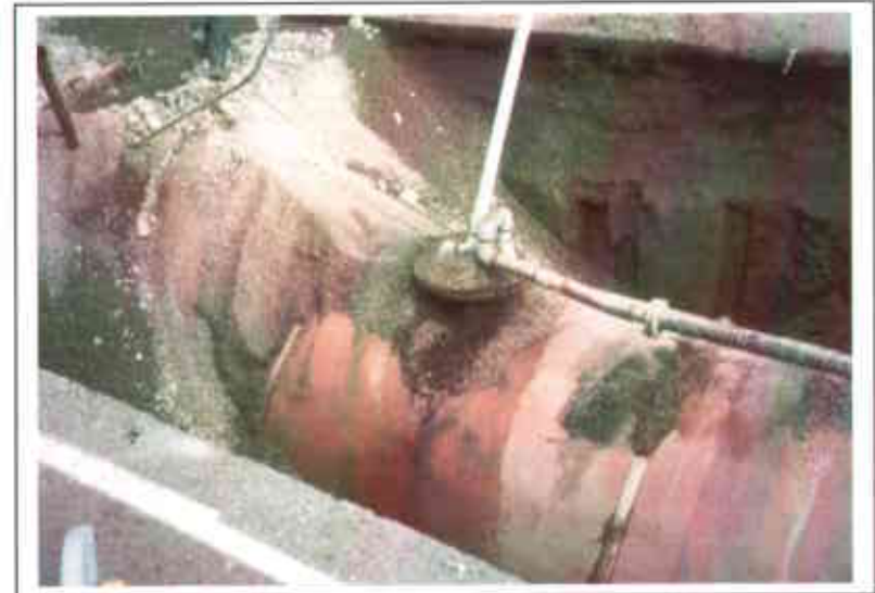
Photo 6. View towards east showing piping and unsealed tank access. Dark stains visible on side of tank due to missing bolts in lid of manhole.
