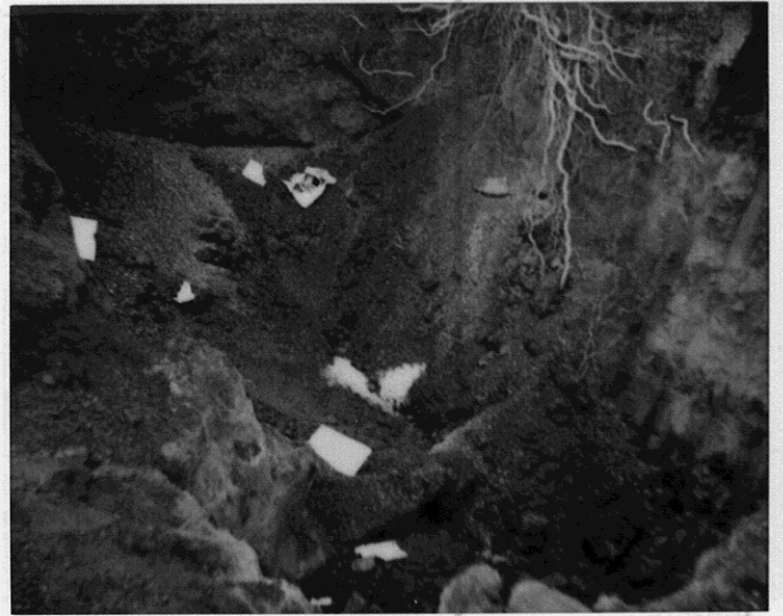
997 Grant Av., San Lorenzo. 12-18-90 Waste oil tank pit bottom immediately after tank removal. 9-10' depth.
