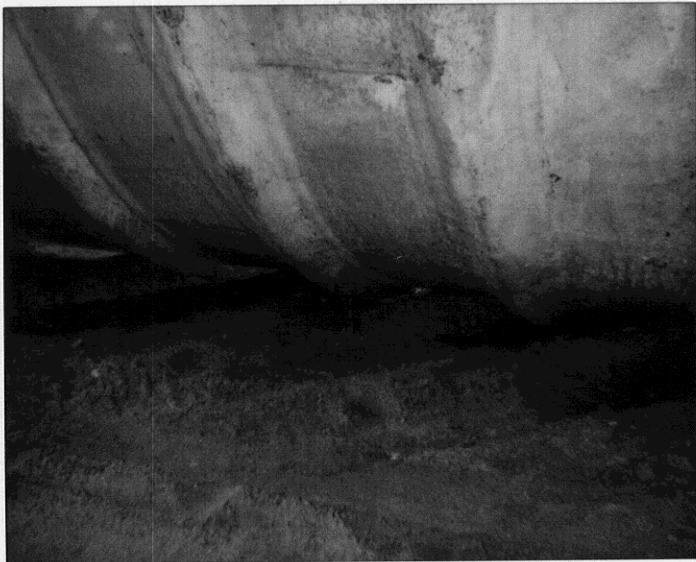
997 Grant Av., San Lorenzo. 12-18-90, middle tank 10k. Far left rib had pin hole to right. Note puddled water.
