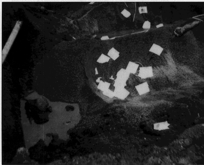
997 Grant Av., San Lorenzo. 12-18-90. Pooled water, w. side of fuel tank pit.
