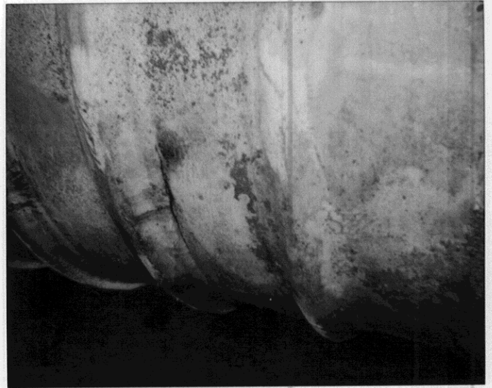
997 Grant Av., San Lorenzo. 12-18-90, middle 10k fuel tank. Crack noted next to rib in center of photo.
