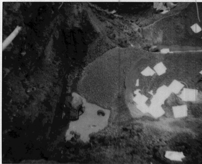
997 Grant Av., San Lorenzo. 12-18-90. Pooled water - w. side of fuel tank pit. Oily sheen present - ~ 11 feet deep.
