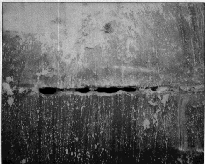
Weyerhaeuser 5" hole in 1000GL tank No. 5570 2-7-91 W. Faulhaber
