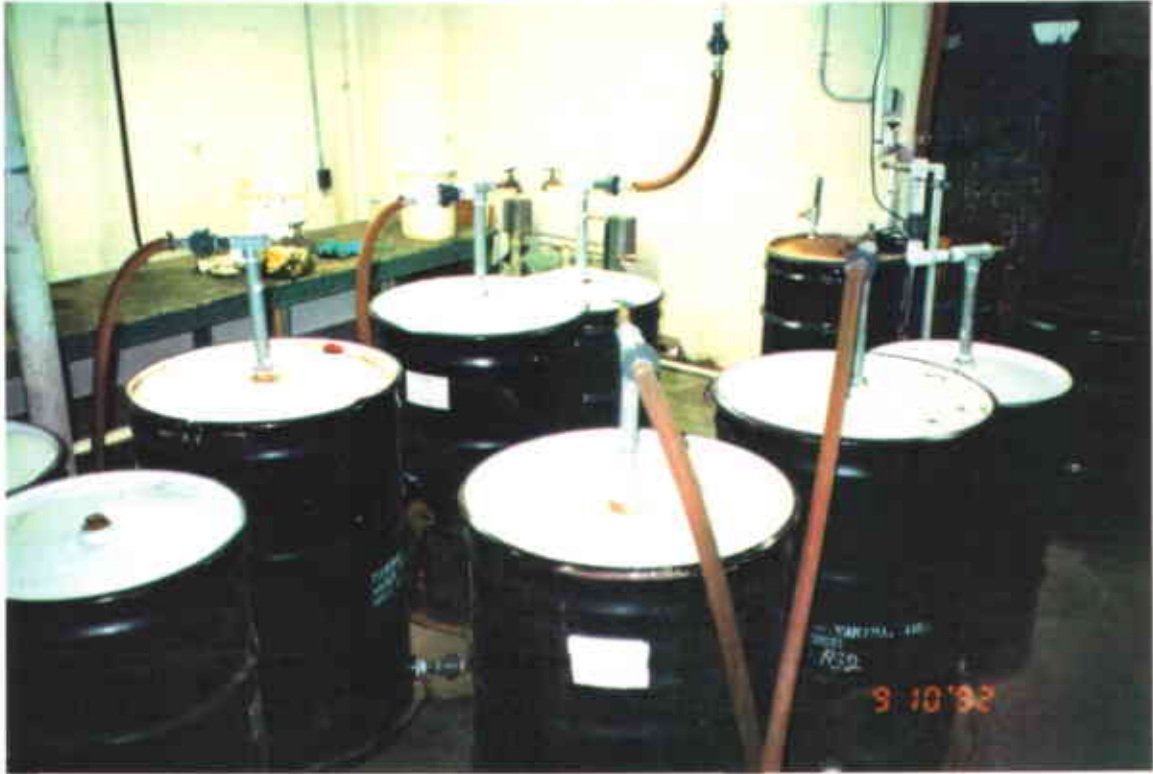
7. Groundwater treating system located inside warehouse, northeast corner of building.
