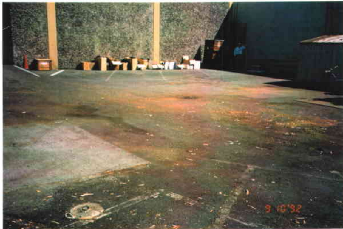
4. Former waste drum storage area located on the west side of the property (facing east).
