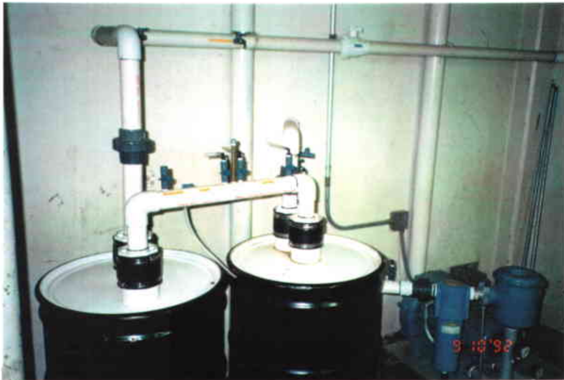
6. Soil vapor treating system located inside the warehouse, northeast corner of building.
