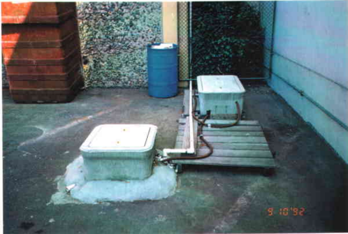
5. Groundwater extraction and pumping system installed in waste drum storage area (Monitoring Well 7), facing east.
