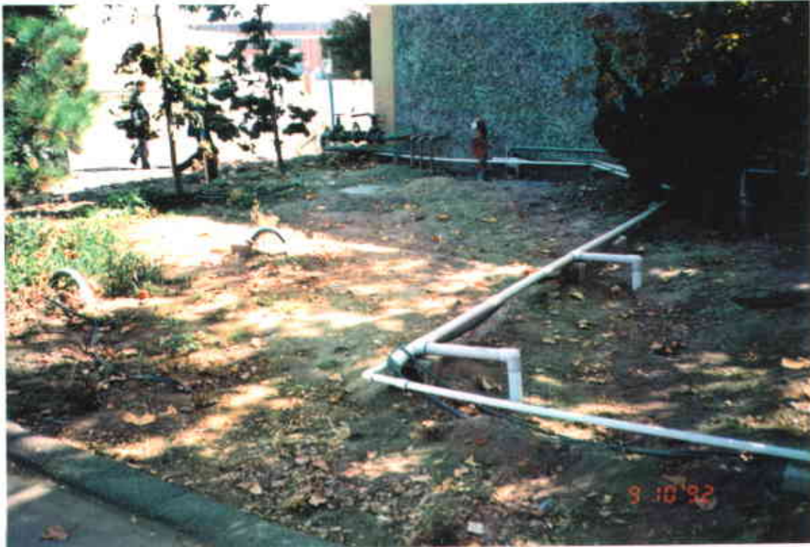
3. Location of excavated methyl ethyl ketone tanks and soil vapor extraction system (facing east).
