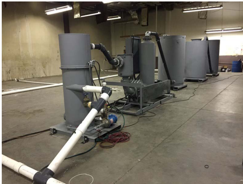
Photo 1. View of SVE equipment. Extracted vapor influent collector pipe (at angle) is plumbed through water knockout tank before blower (at center), then through the three treatment vessels (right side of photo).
