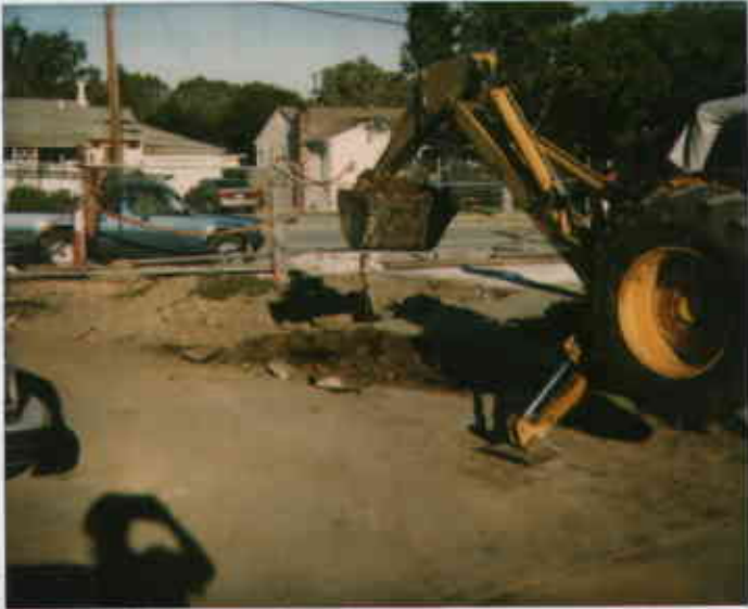
508 E. Lewelling Product piping on east side of former tank pit
