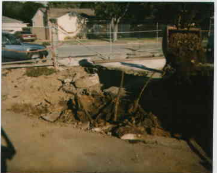
508 E Lowelling Product piping on east side of tank pit. (Two parallel to one another) 054183331173-2 5792 0138 9/15/84 Juliet Shinn
