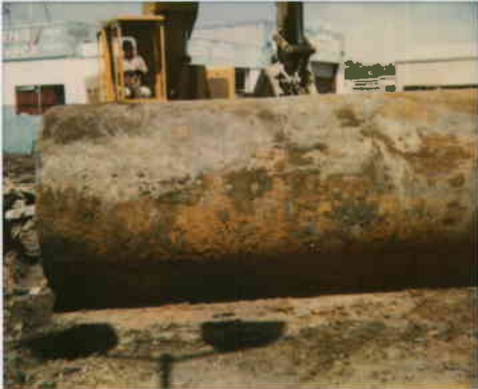
508 E. Leavelle Blvd, S.L. 8/26/73 2nd 2,000-gallon gas UST. Corrosion but no holes noted. 03317211124-2 Tubert Shure
