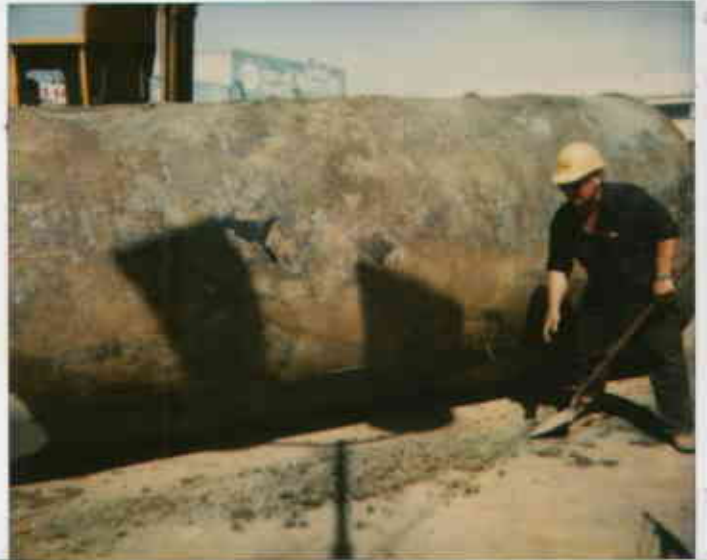
508 E-Leavelle Blvd., S.L. 8/26/73 4,000-gallon 03317211124-2 and 4 pin-size holes. Corrosion, putting Tubert Shure
