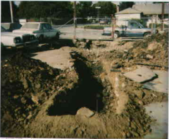
508 E Lowelling Product piping trench on east side of tank pit. Parker (blue/black) clayey soil (appears native). Slight odor in areas of this clay. 054183331173-2 5787 0138 t/15/84 Juliet Shinn
