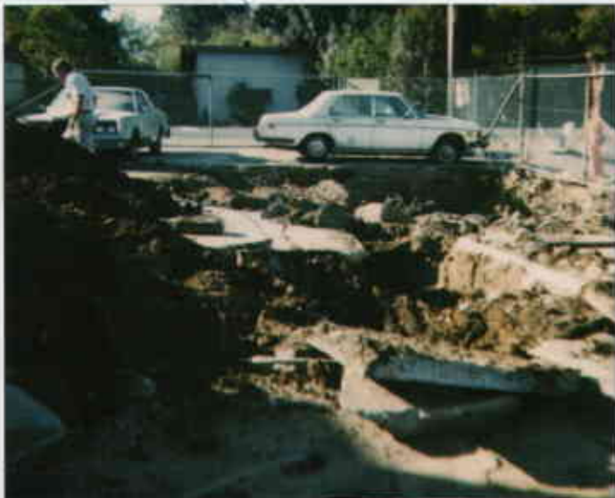
508 E. Lewelling Tank pit in background trench on north of pit & former dispenser location in foreground.
