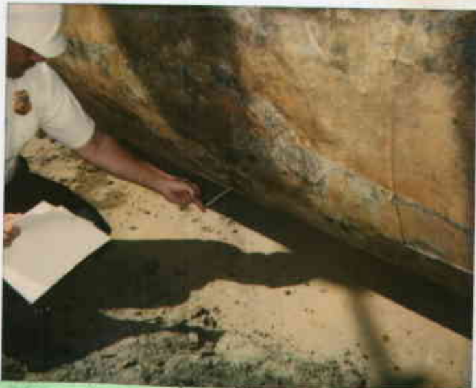
508 E. Lowelling Blvd., San Lorenzo 8/26/93 83317211124-2 Pen-size hole in 4,000-gallon gas UST. Juliet Sher
