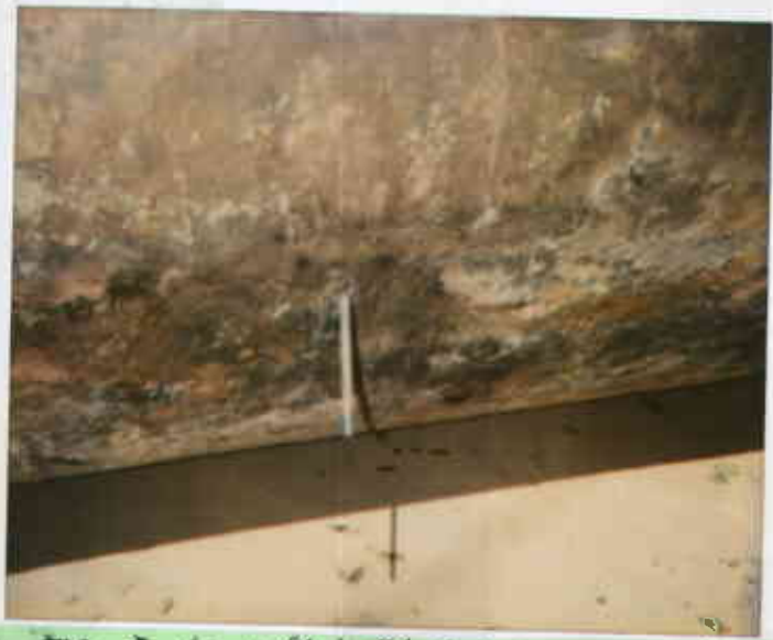
508 E. Lowelling Blvd, S.L. 8/26/93 Pen-size hole in bottom of 4,000-gallon UST. 83317211124-2 Juliet Sher
