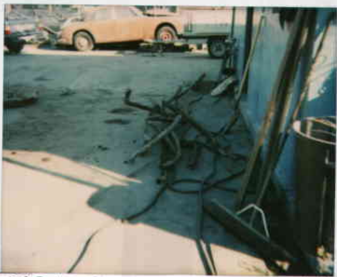
508 E Lowelling Sum total of product piping removed from both the east & north side of former gas tank pit. 054183331173-2 5783 0138 9/15/84 Juliet Shinn
