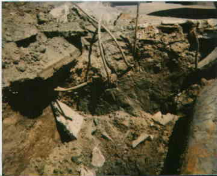
508 E. Leavelle Blvd, S.L. 8/26/73 Stained soil observed on east wall + floor of pit 03317211124-2 of pit where 2,000-gallon UST was. (on the end of pit) Tubert Shure
