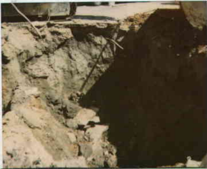
508 E. Lewelling Blvd, S.L. 8/26/93 Stained soil on east, south, north walls of pit and bottom for 4,000-gallon gas tank. 83317211124-2 Julius Stein
