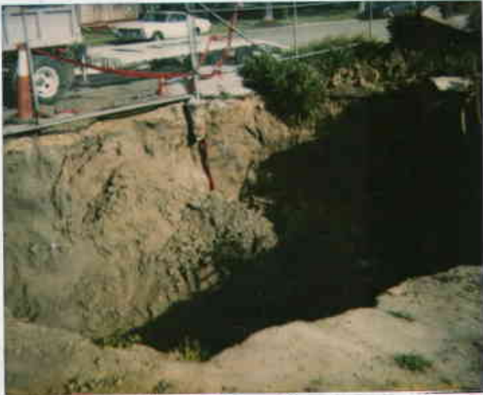
508 E. Lawelling, San Lorenzo 4/14/99 Tank pit where over 4,000 gallons of 2 3,000-gallon gas USTs used to 09318221467-2 be. Max excavated some 0547 1730 material since the pull. Juliet Shinn
