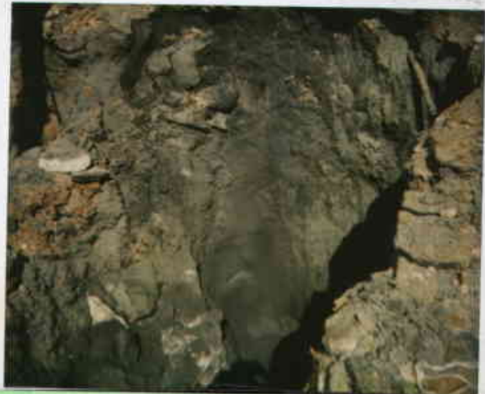
508 E. Lowelling Blvd, S.L. 8/26/93 83317211124-2 Found sand underneath 4,000-gallon gas UST. Juliet Sher
