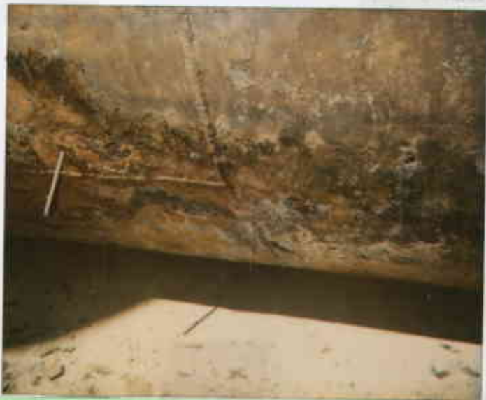
508 E. Lowelling, S.L. 8/26/93 83317211124-2 Several pen-size holes in bottom of 4,000-gallon UST. Juliet Sher
