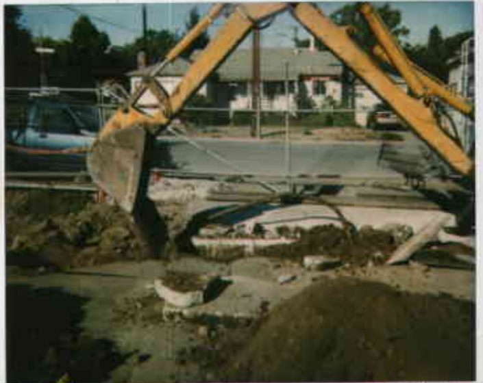
508 E. Lewelling Product piping leading to former dispenser on north side of former tank pit. (Two alongside one another)
