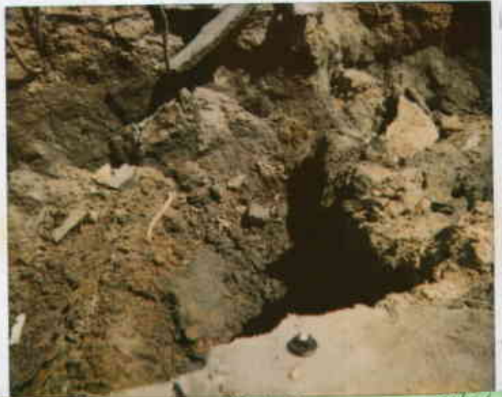
508 E. Lewelling Blvd, S.L. 8/26/93 Stained soil at bottom & east sidewalk of tank pit 83317211124-2 for 2nd 2,000-gallon OST. Julius Stein
