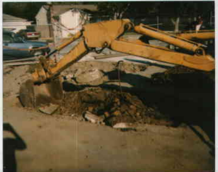
508 E. Lewelling Product piping trench east of the former tank pit. (Two parallel to one another). Some odor noted in darker clayey material in trench.
