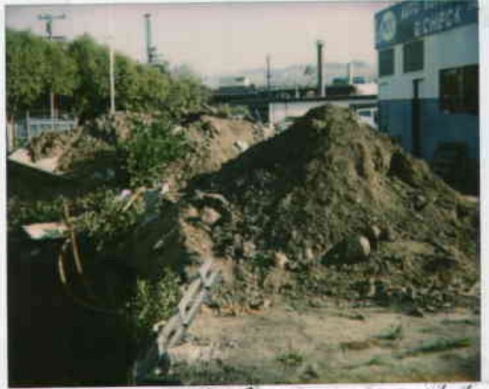
508 E. Lawelling, San Lorenzo 4/14/99 Stacked soil was not 09318221467-2 covered when I arrived 0547 1730 out on site. Juliet Shinn
