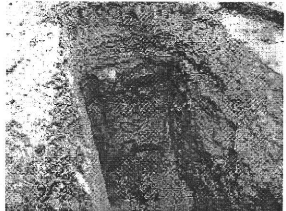
#8 Western end of GAIA TP-6. 3-inch size drain rock encountered at 6.5 feet bgs.
