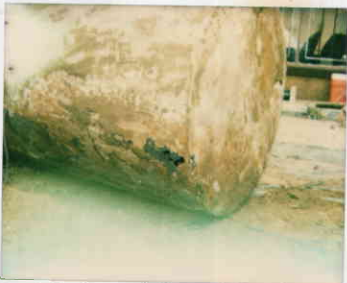
Tank H large hole in 500-gal gas UST. Lim/Former Exxon, 250-8th St, Oak 94607 5-7-92 JEberle
