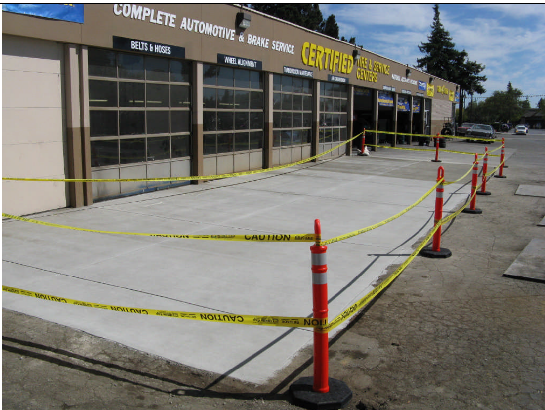
View of the Site after the completion of excavation activities and concrete restoration.
