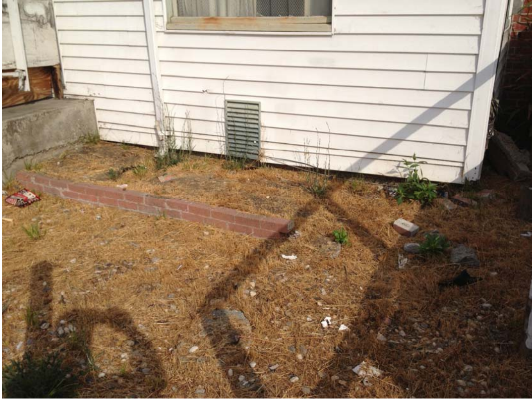
Plate 1. Property located next to site on 152 nd St., showing crawl space underneath house
