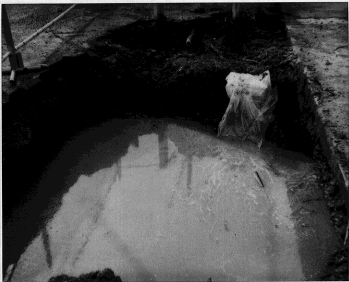
CAMP PARKS 1-550 Diesel 2/23/93 Water in pit Jeff
