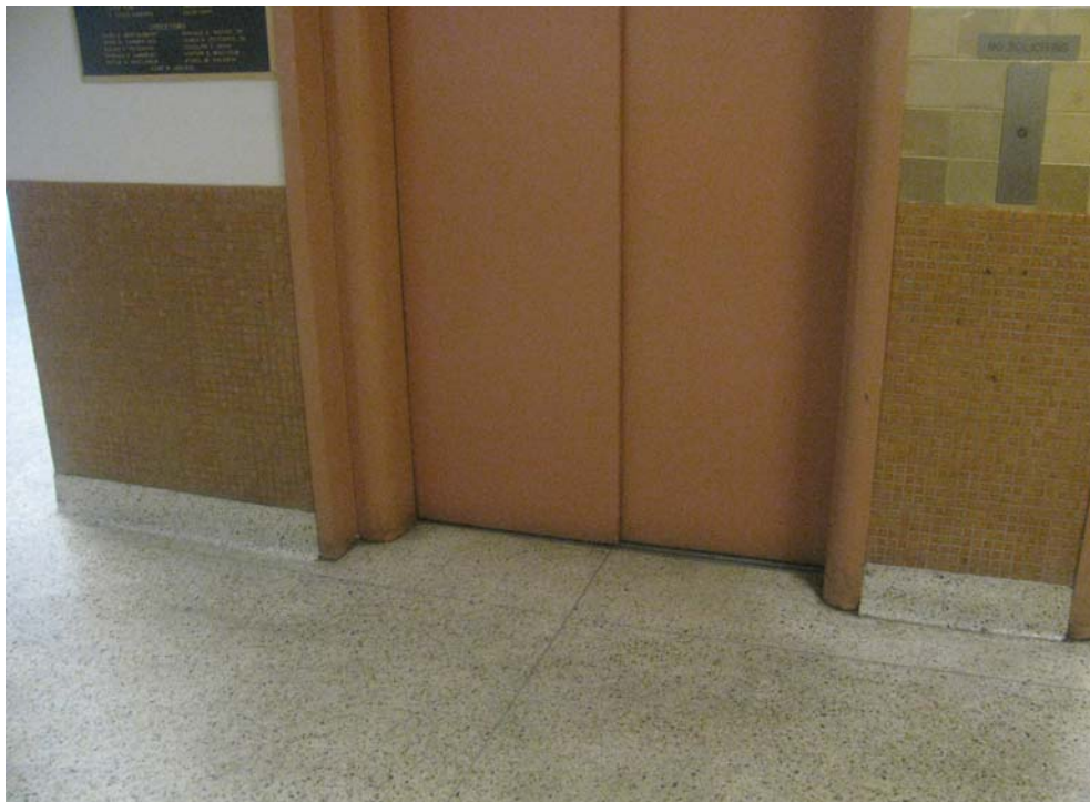
Plate 2. View of second elevator car, door closed
