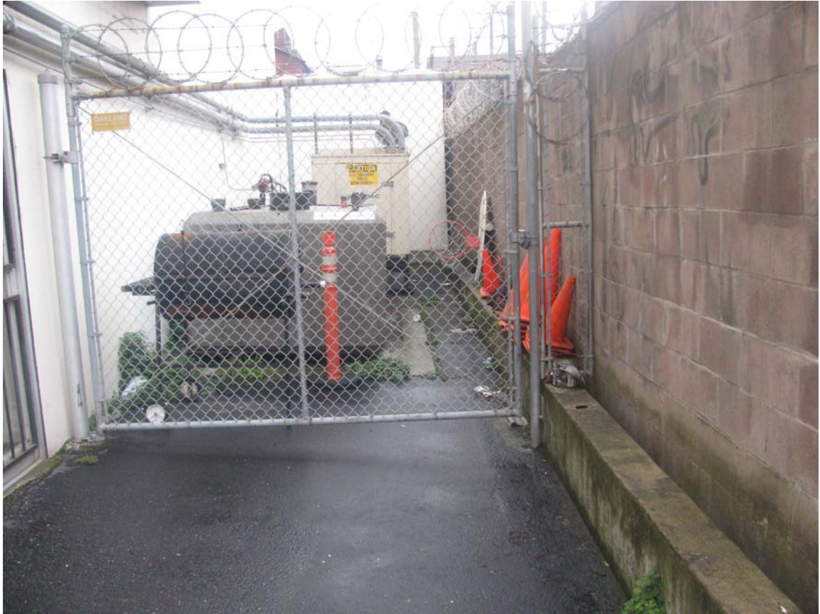
Plate 14. Generator and fuel storage tank southeast corner of Red Cross building, near rear entrance of Red Cross, parking lot side
