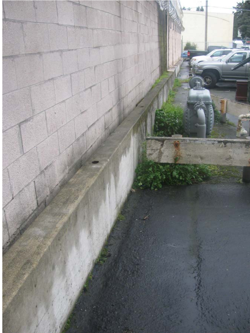
Plate 16. Retaining wall and wall, boundary with Glovatorium and Red Cross parking lot, towards Manila ave.
