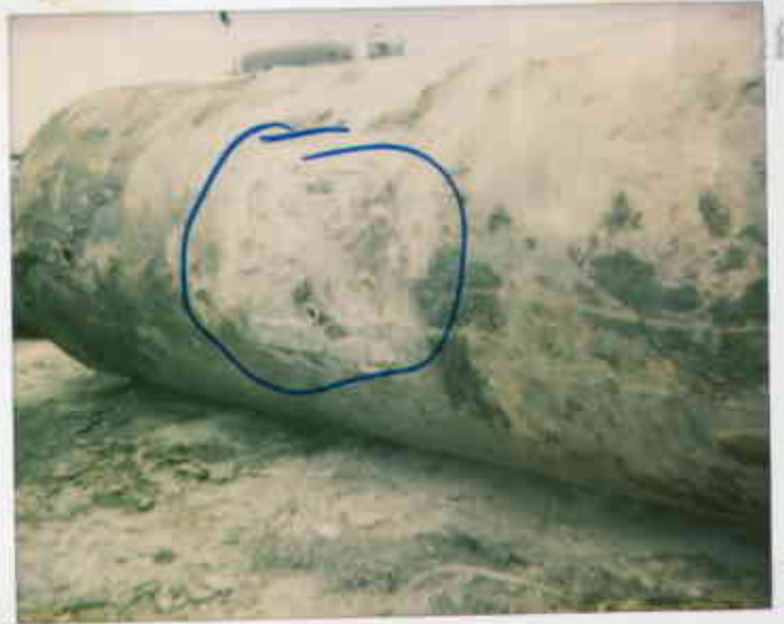
Tank C - welded top 5/18/94 ST10567
