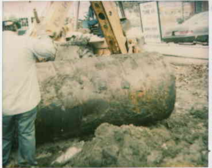
5/18/94 Waste oil tank (ST06)
