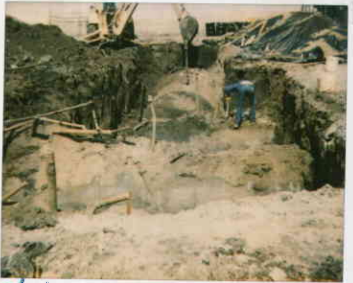
5/18/94 ST10567 Gasoline tanks common area.
