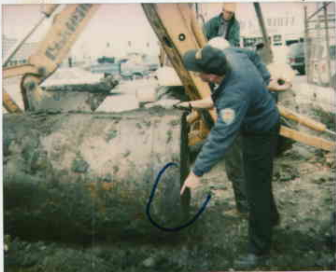
5/18/94 ST10 567 Waste oil tank rd hole
