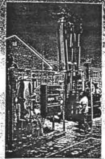
A 30 GPM service station, GAC Fluid Bed package plant.
