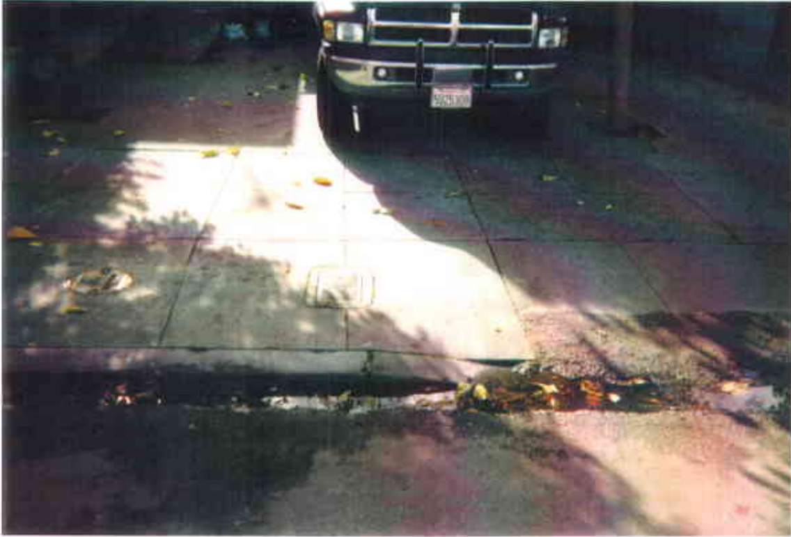
9. Water meter vault box along east property boundary
