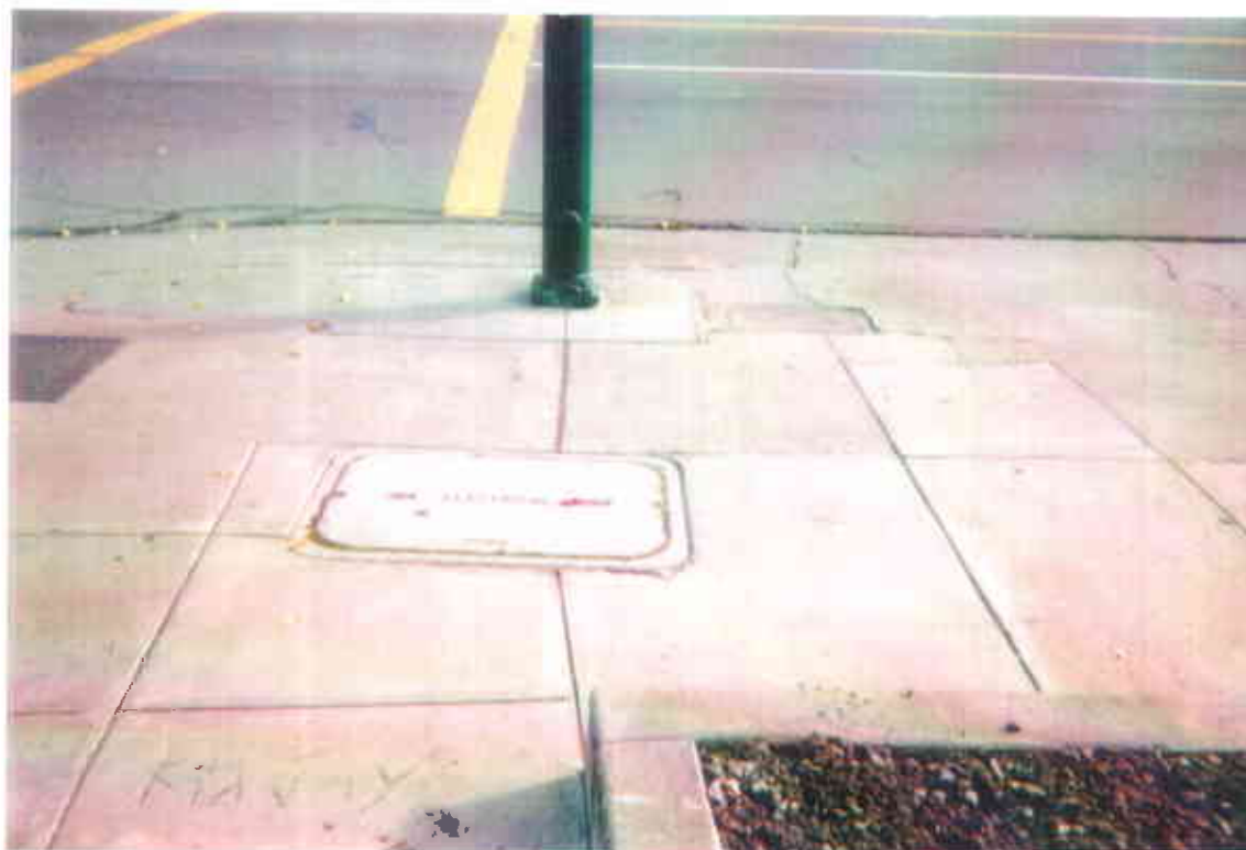
12. Electrical utility box located along south property boundary
