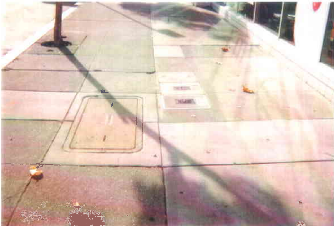
14. PG&E and Pacific Bell vault boxes located near southwest corner of site.
