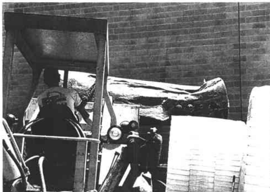
PHOTO 6: UST showing area of rupture near vent pipes created during UST removal.
