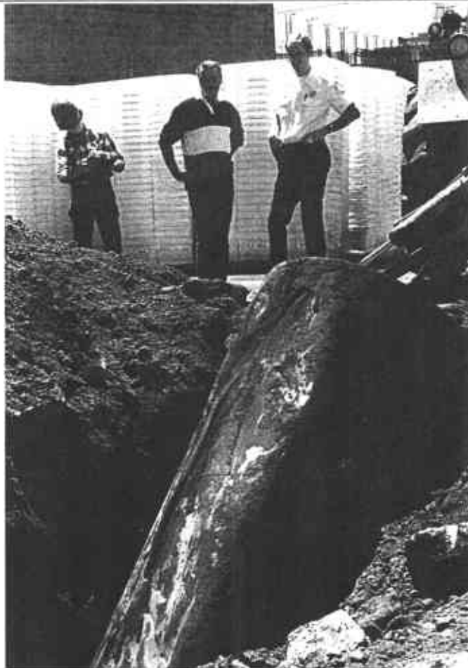
PHOTO 3: Upending of tank in excavation: Some breakage of tank occurred during removal.
