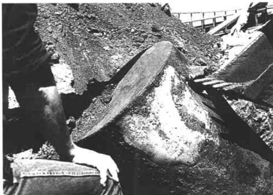
PHOTO 4: Close-up of rupture created during removal.
