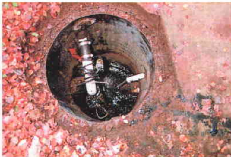
SUMP WITH PUMP AND INFLOW PIPE
