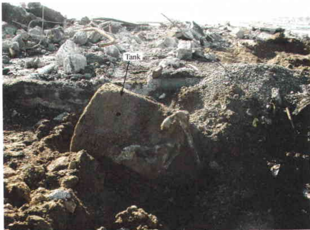
Photograph 4: 100-gallon underground storage tank discovered during foundation removal of Building 301 (looking west).
