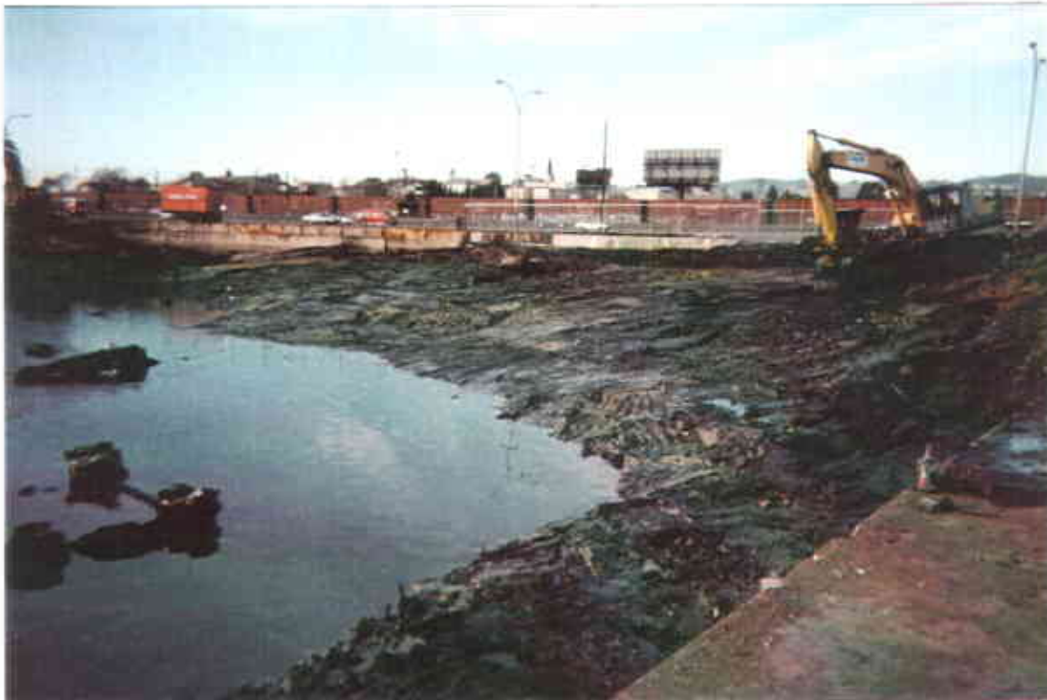
6. Photograph showing sandblast grit and debris supra-tidal zone area after removal activities
