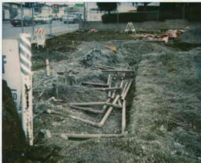
3530 MacArthur 4/26/94 Gas product piping in trench. Broken up during excav. Rinsed 09318221467-2 0547 1737 Subject Site
