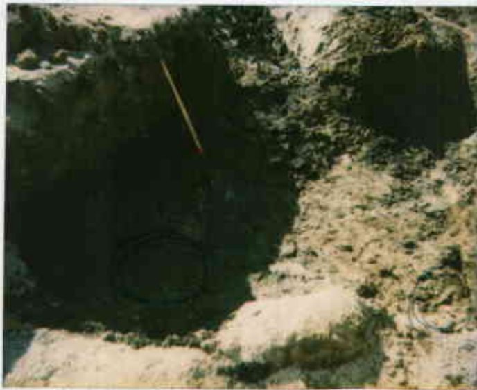
3530 MacArthur Oakland 5/2/94 The circled areas are sample locations PX-2 thru PX-5 in overexcavated piping trench. 09318221467-2 4547 1721 Juliet Shinn
