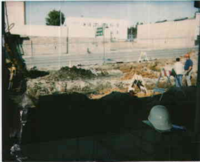
3530 MacArthur Oakland 5/2/94 Overview of site & piping trenches taken from inside building. 09318221467-2 4547 1721 Juliet Shinn
