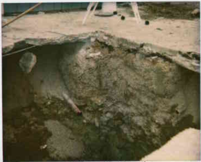
3530 MacArthur, Oakland 5/24/99 12215117976-B The first pipe did not appear to be sealed & capped or reused. Juliet Shui
