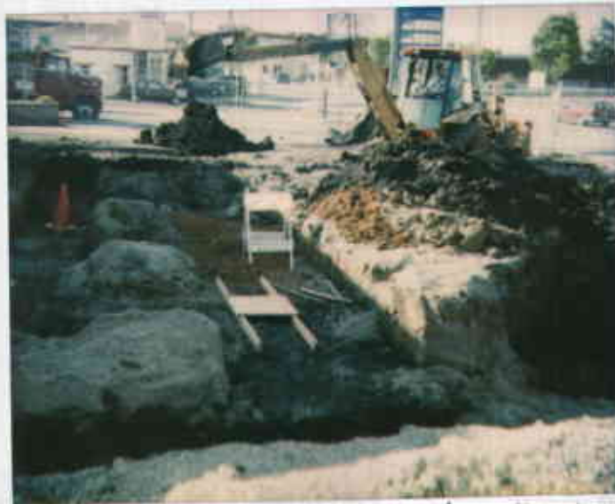
3530 MacArthur, Oakland 5/2/94 Primary overexcavation area is to the extreme right and they well we skimming more soil from the trench for lower depth piping, in center of picture 09318221467-2 0547 1732 Juliet Shinn
