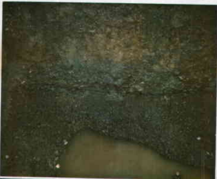
3530 MacArthur, Oakland 5/19/74 12215117976-B Stained soil observed along all four sidewalls of 1,000-gallon waste oil UST. Juliet Shen
