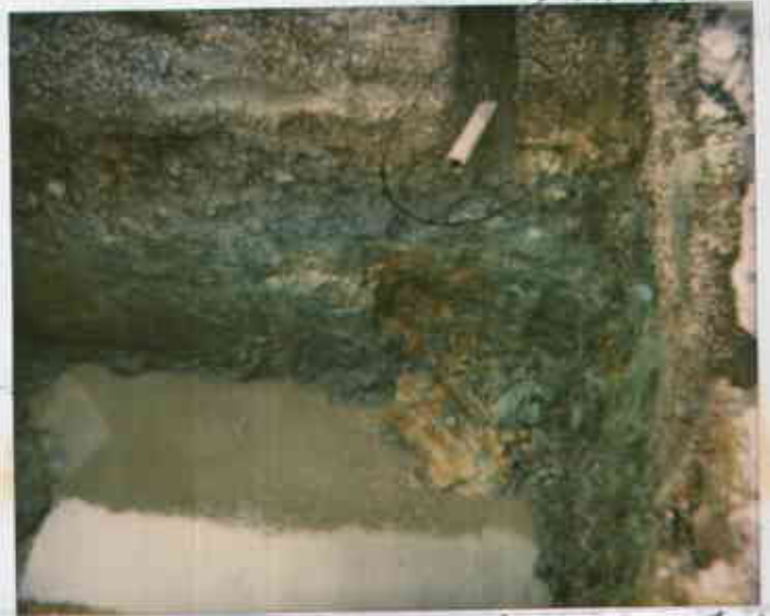
3530 MacArthur, Oakland 5/19/74 12215117976-B Waste oil UST pit w/ stained soil Soil sample collected from beneath fill pipe. Juliet Shen
