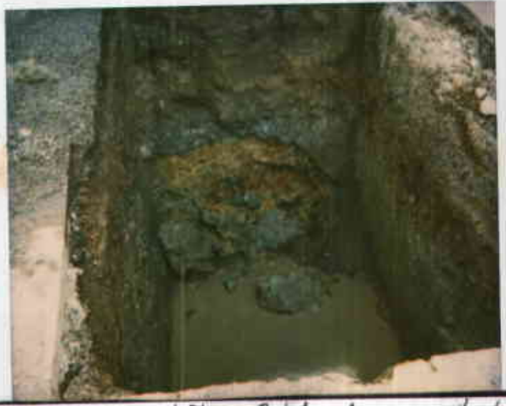
3530 MacArthur, Oakland 5/19/74 12215117976-B Stained soil on south wall of pit (waste oil UST pit). Juliet Shen
