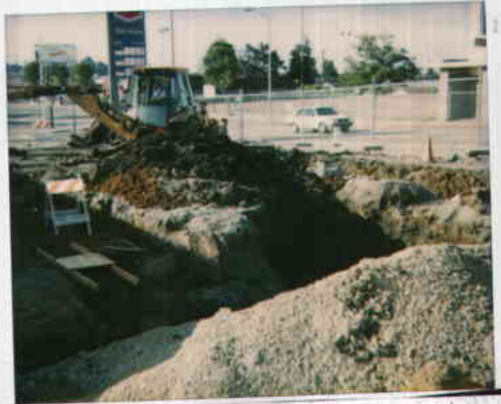
3530 MacArthur, Oakland 5/2/94 Area of overexcavation, in westernmost former piping trench where 1200 ppm gas was initially identified. 09318221467-2 0547 1732 Juliet Shinn
