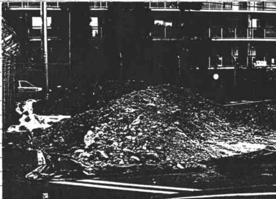
CONTAMINATED SOIL STOCKPILED BEHIND BUILDING
