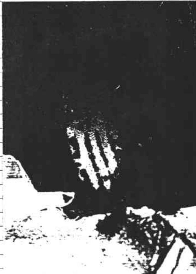
GROUNDWATER WITH FLOATING PRODUCT IN TANK D EXCAVATION
