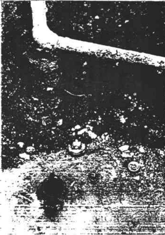
TANK B CORRODED FILL PIPE
