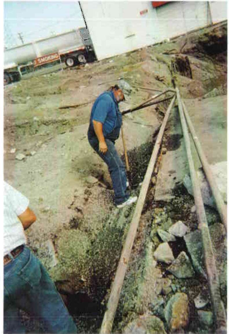
H) View of product lines south of tank cavity.
