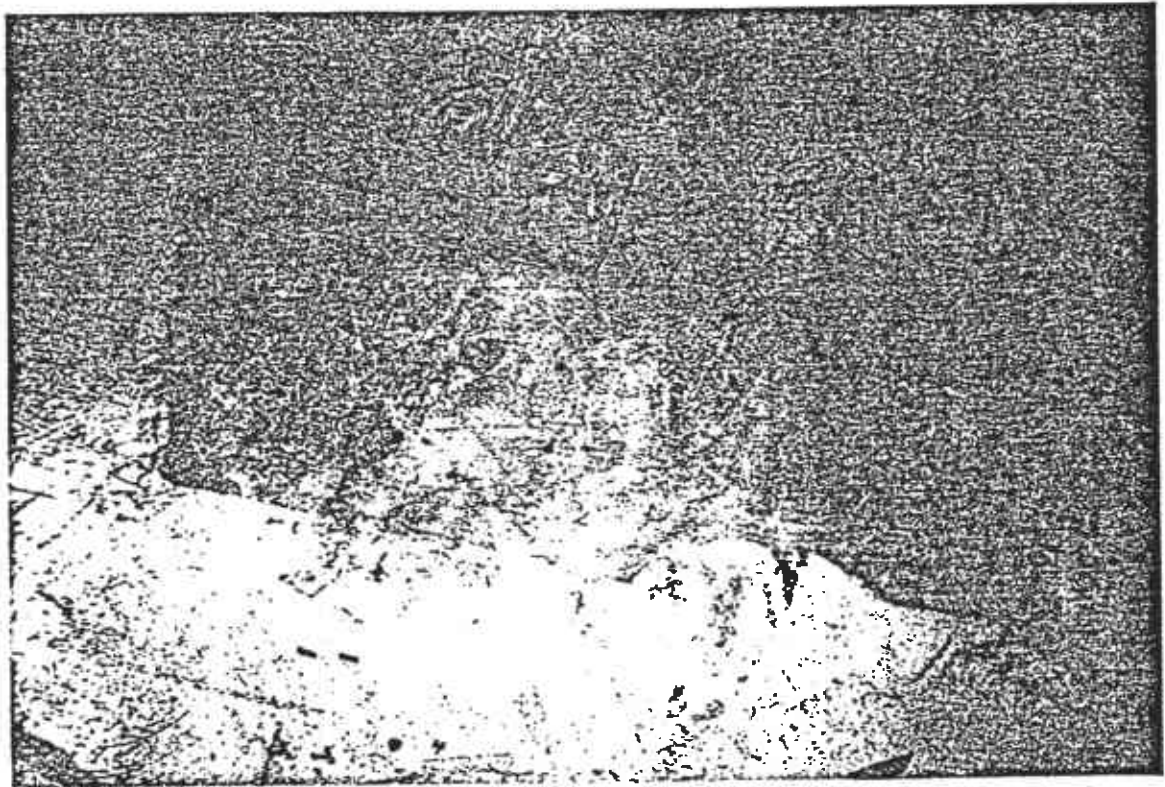
Photo 24 - Bare patch of concrete in west drum storage area. Probable cause is spill or leak from drum of new immersion cleaner which completely dissolves the epoxy coating.
