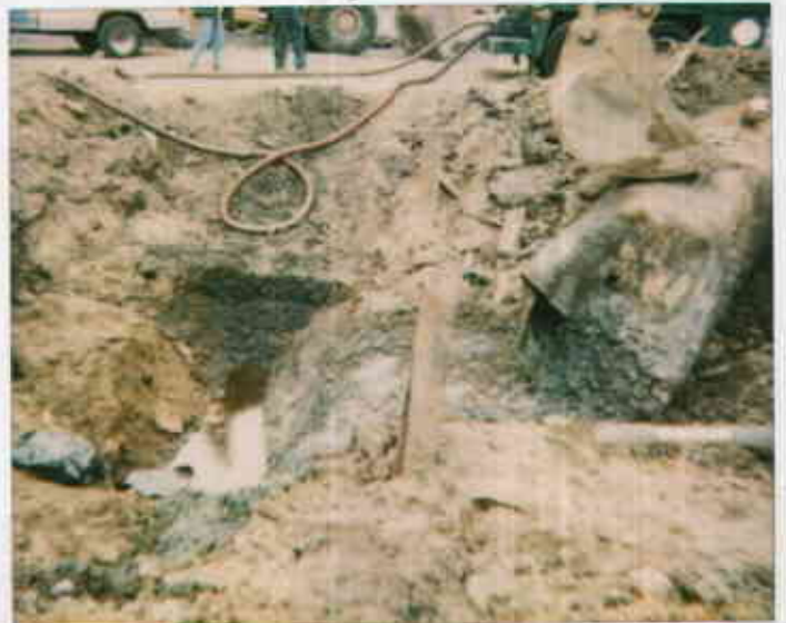
6/2/95 08416201510-2 P.C.C. 2026 5835 - damaged end 501 5th Ave, water in pit obv. con tank started of tank
