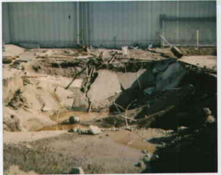
PCC 11/4/93 333 E 8 th Caved-in pit w/ mucky G.W.
