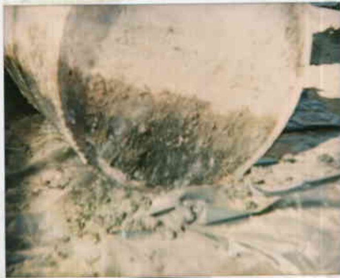
054163023672W 6/21/95 0539 8964 end of 500 tank, water leaking
