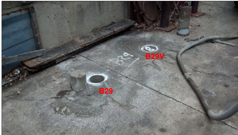
Photograph No. 5 – North view of rear concrete-paved storage yard, showing locations of Borings B29 & B29V following concrete coring (8"-Dia.) activities; B29V located approximately 3 feet northeast of B29 (GGTR, Nov. 2015).
