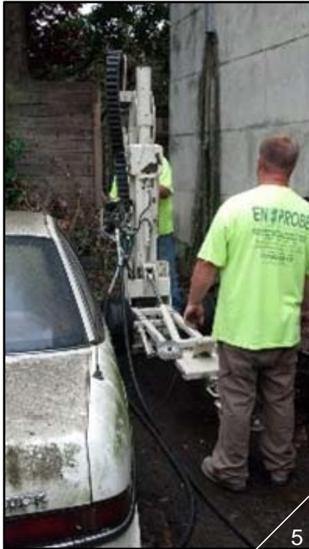
Photograph No. 4 – Southwest view of rear concrete-paved storage yard, showing EnProbe representative concrete coring at B26 in vicinity of subsurface sanitary service lateral cleanout and oil/water separator (GGE, August 2013).
