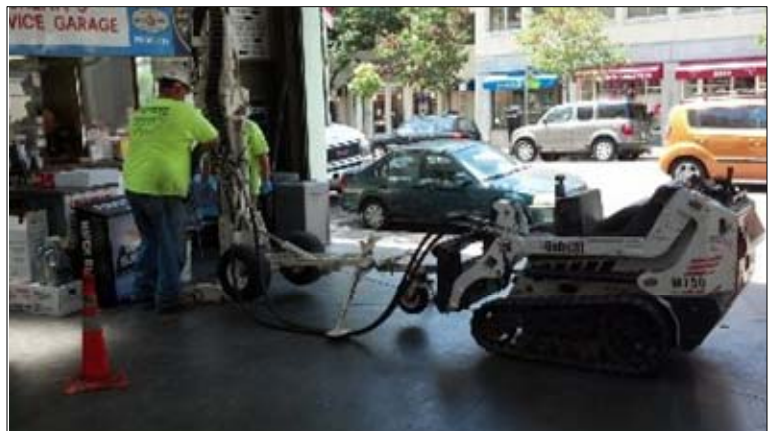
Photograph No. 6 – Southwest view of interior service garage area, showing EnProbe representatives drilling for discrete soil sampling and installation of soil gas probe, SG-2 (GGE August 2013).
