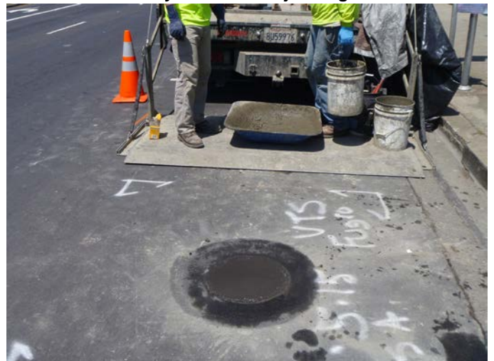
Monitoring wells patched with concrete and black dye to match adjacent grade
